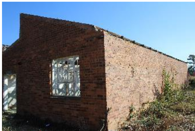
Figure 23: Exterior of Site Complex 4. Note the broken windows
