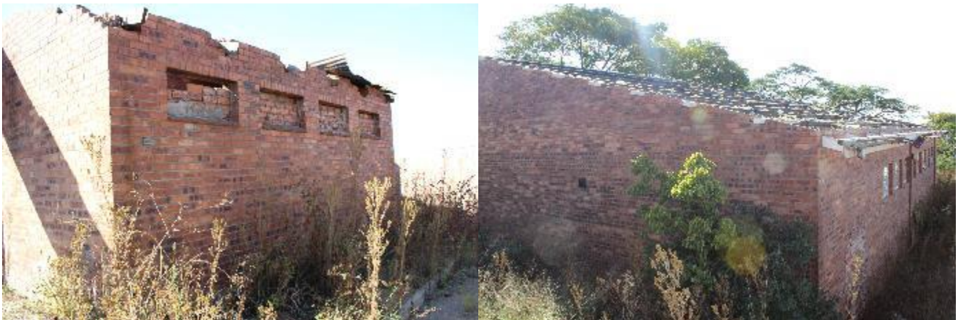
Figure 14: Ruins of Site Complex 2. Note that the buildings do not have any windows or roofs.
