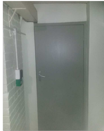
Photo 4.6.25: Passage 2 – Timber door to adjacent plant room with biometric control
