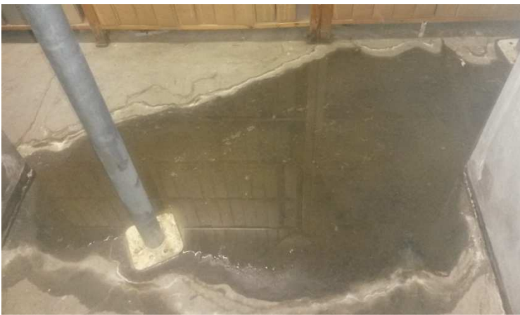
Photo 4.6.3: Standing water inside basement next to existing prop
