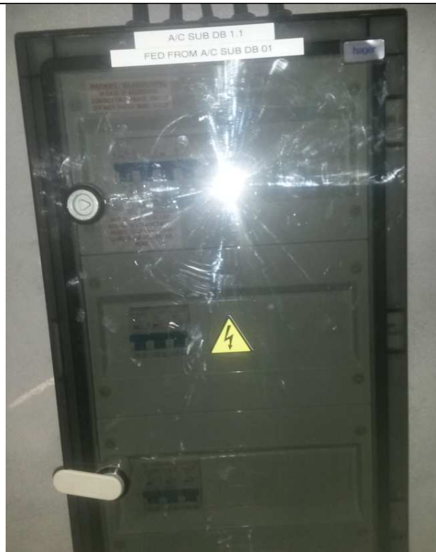
Photo 4.6.26: Basement - Sub DB at Passage 3 doorway
