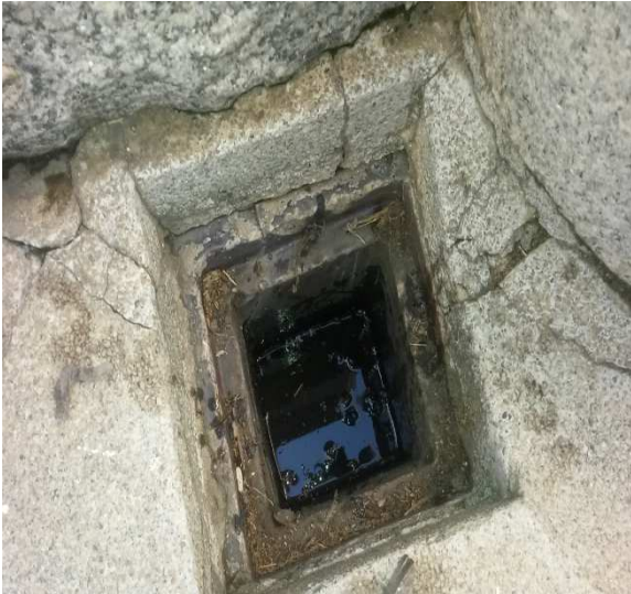
Photo 4.6.7: Blocked storm water drain at bottom of steps
