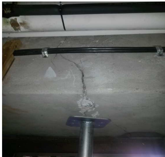
Photo 4.3.2: Vertical cracks through down stand beam, following line of crack through slab
