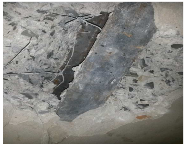
Photo 4.2.8: Another steel beam with little to no corrosion some with reinforcing mesh visible
