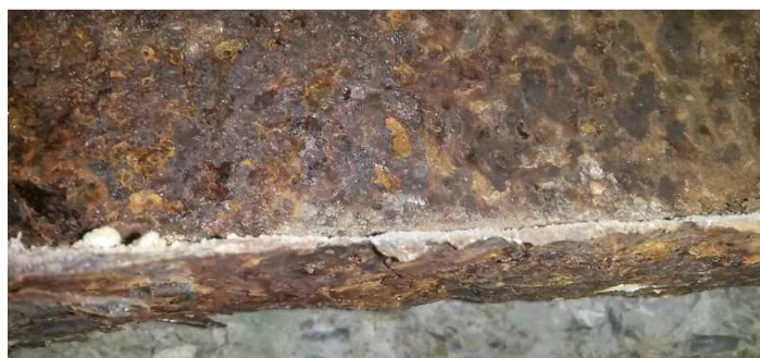
Photo 4.4.8: Bottom flange of beam that has extensive pitting corrosion (1-2mm rusted material remaining)
