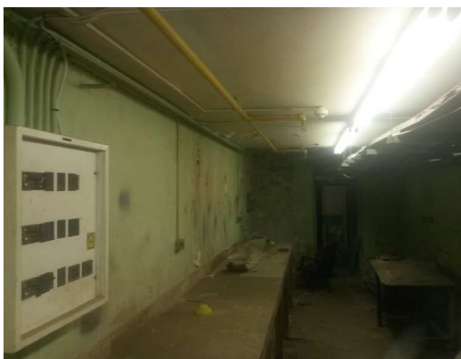
Photo 4.6.20: Passage 2 - Internal Distribution board at far end of basement corridor
