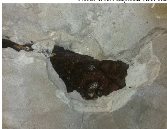
Photo 4.4.4: Exposed steel beam with severe surface corrosion visible
