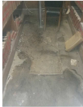
Photo 4.6.4: Water mark from previous water leak elsewhere in basement
