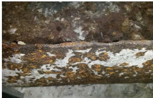
Photo 4.4.7: Bottom flange of beam that has extensive surface corrosion (+/- 4mm thick steel remaining)
