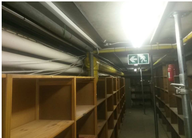
Photo 4.6.14: Passage 3 – View towards Passage 2 door - Yellow fire water line entering and exiting the passage with fire escape signage
