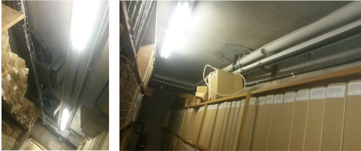
Photo 4.5.33 & 34: Overhead services closer to entrance of basement ( far left corner)
