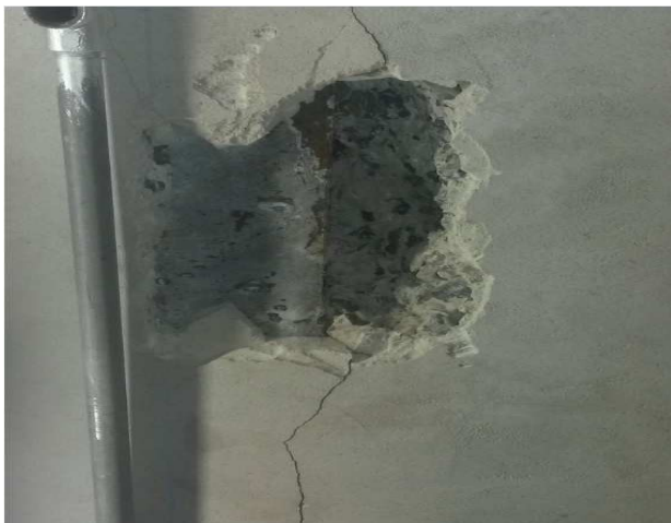
Photo 4.2.7: Crack in slab with bottom flange of steel beam visible, no visible corrosion
