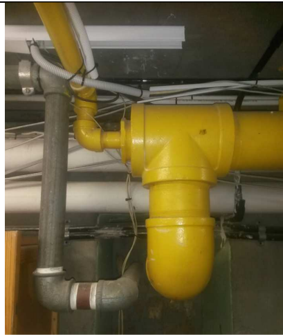
Photo 4.6.13: Fire water system reducer and other services
