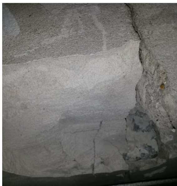
Photo 4.5.2 More blows - Large portion of plaster broke off
