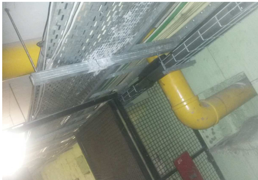
Photo 4.6.19: Passage 2 - Yellow fire water line exiting basement with cable tray below
