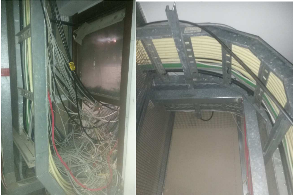
Photo 4.5.38 & 39: Numerous electrical cables entering the basement at the near left corner of the basement
