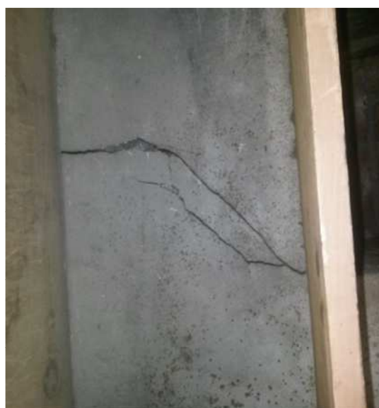
Photo 4.5.9: Horizontal crack in wall element next to plant room of Assembly chamber
