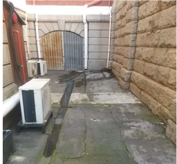
Photo 4.6.8: Blocked drain at back corner of balcony
