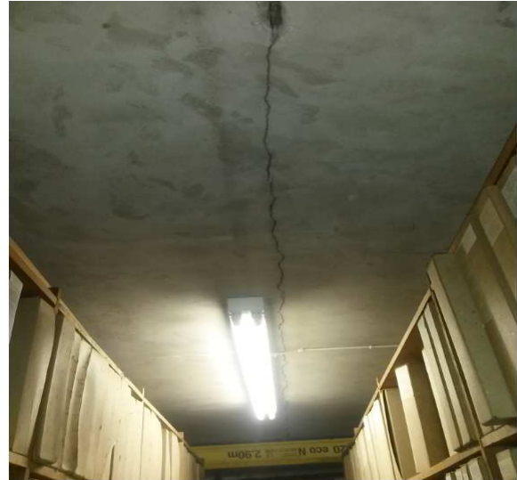
Photo 4.2.2: Typical cracks in plastered finish of slab overhead
