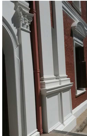
Photo 4.6.2: Rainwater downpipe going into staircase structure, probably resulting in observed corrosion due to water leaking out from encased pipe.
