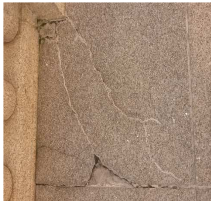
Photo 4.6.6: Damaged granite panel on balcony
