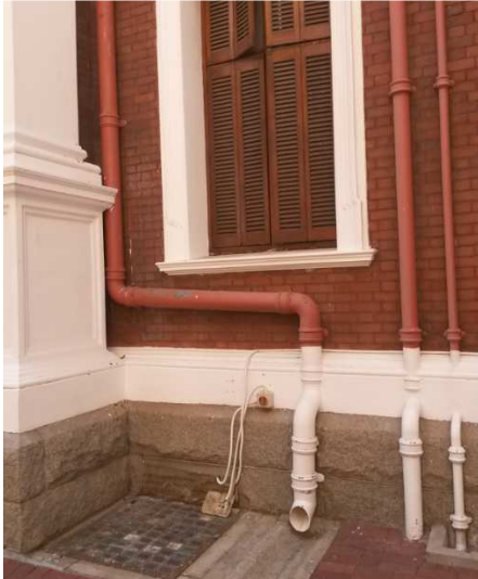
Photo 4.6.13: Rain water downpipe on other side of building Where stormwater is diverted via a surface channel.
