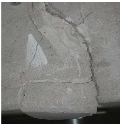
Photo 4.5.1: Crack in beam that is propped, after a couple of blows with a hammer – some small cracks formed
