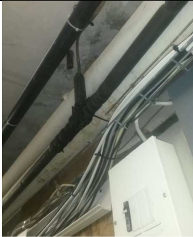
Photo 4.6.2: Overhead Mechanical services where water is leaking from
