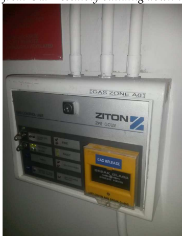
Photo 4.6.8: Gas Control Unit on outside of basement entrance door
