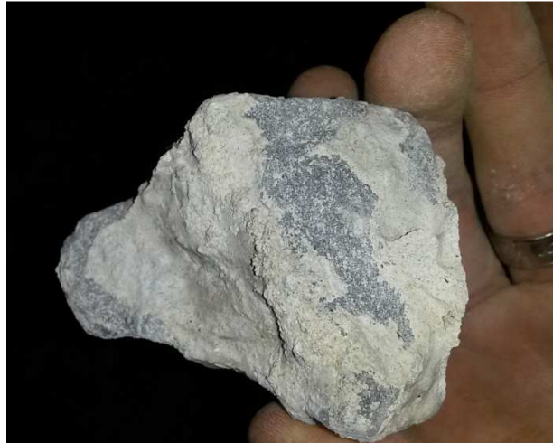
Photo 4.5.7 Aggregate size of 75mm was used during construction of the beams. Modern day concrete used in concrete beams is made up of 19mm stone. 75mm aggregate is normally only used in mass concrete fill underneath foundations.
