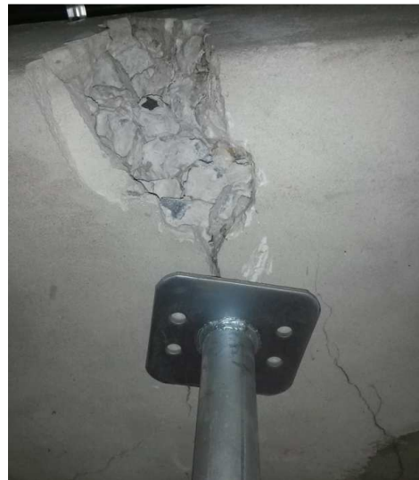
Photo 4.5.5 No more blows – size of exposed beam visible from below
