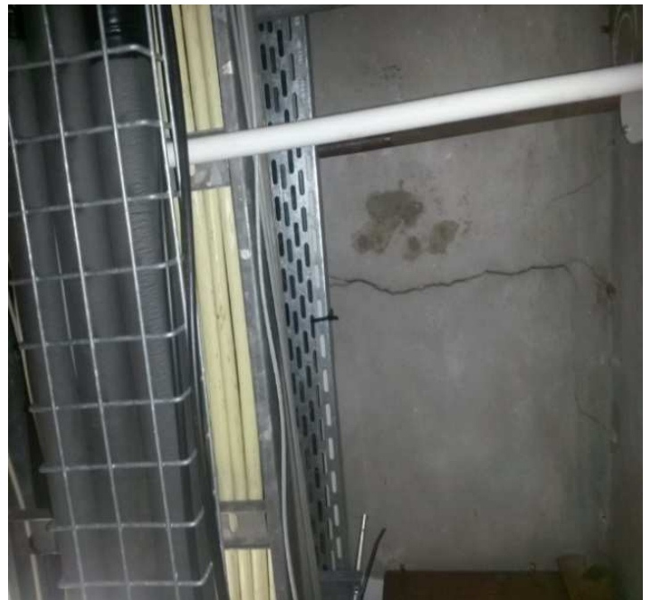
Photo 4.2.4: Services in cable trays with cracks in floor above
