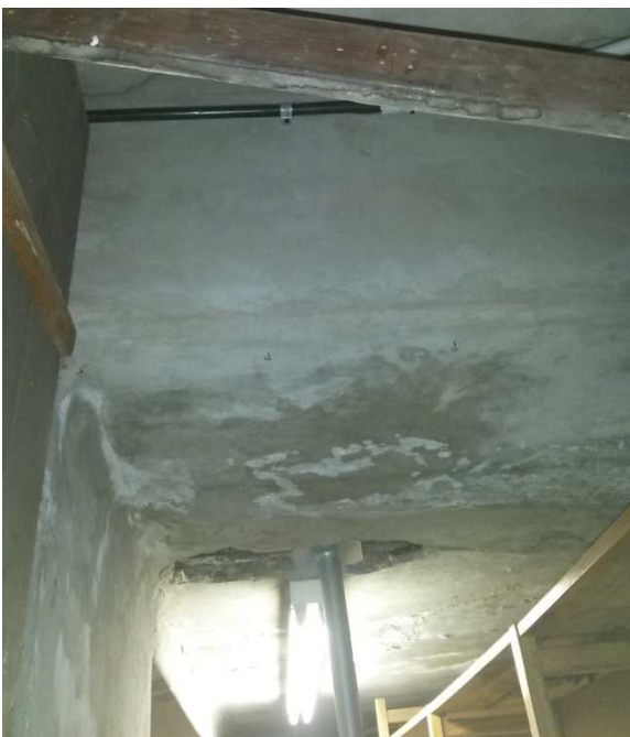
Photo 4.2.3: Portion of slab against far wall below outside balcony that is 500mm lower than rest of the slab
