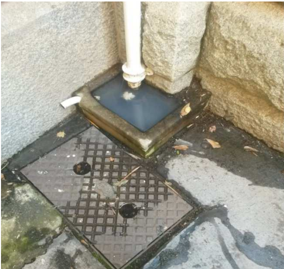
Photo 4.6.9: Close-up of blocked drain
