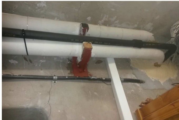
Photo 4.5.35: Overhead services with cracks in beam visible
