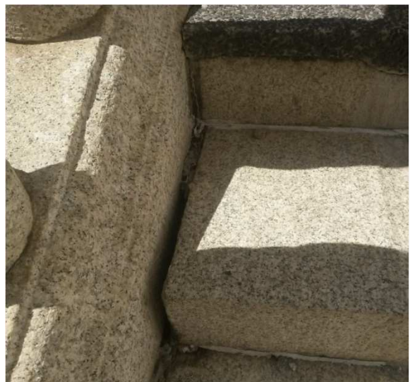
Photo 4.6.4: Joint sealing damaged on edges of granite step
