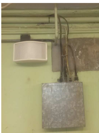
Photo 4.6.21: Passage 2 - Services inside of basement
