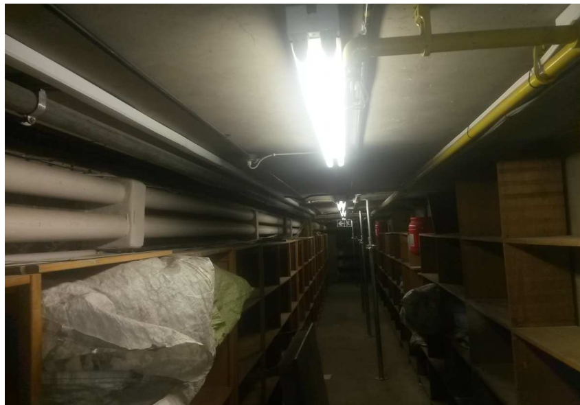
Photo 4.6.15: Passage 3 – View with basement door behind. Note fire suppression units
