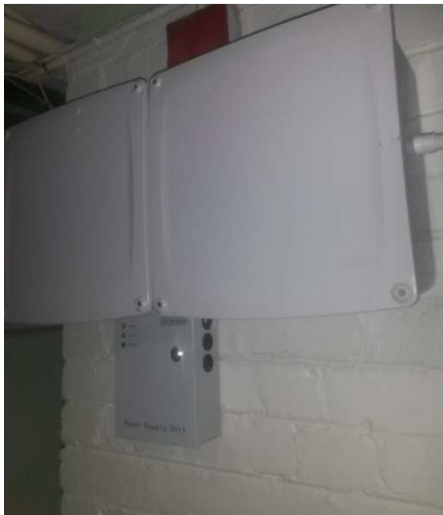
Photo 4.6.24: Passage 2 - Security related services just outside basement passage
