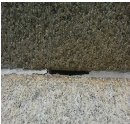
Photo 4.6.5: Joints between steps with visible gaps
