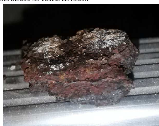
Photo 4.4.5: Portion of corrosion chipped off of beam
