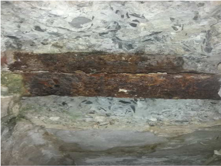
Photo 4.2.5: Steel beam inside concrete floor that is severely corroded
