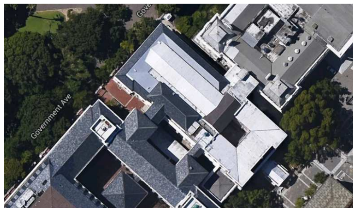
Photo 1.2: Close up aerial photo of Old Assembly building, at the Parliamentary Precinct
