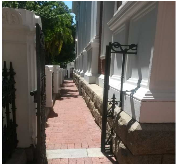
Photo 4.6.10: Side of building on Government Avenue with rainwater down pipes going underground next to granite cladding
