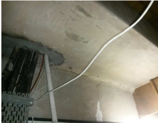
Photo 4.3.1: Crack along slab/beam interface
