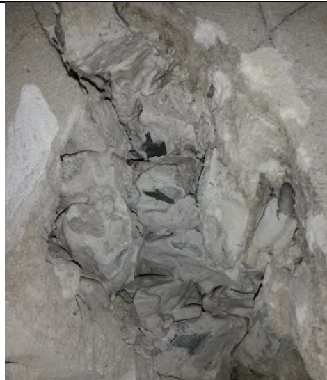
Photo 4.5.4 More blows – some of the aggregate falls out, with no visible reinforcing steel in the beams
