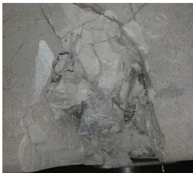
Photo 4.5.3 More blows – Plaster fell off exposing some large aggregate covered with a some intermediate cement
