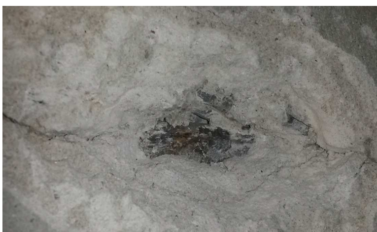
Photo 4.4.2: Another Exposed Steel beam with slight surface discoloration visible
