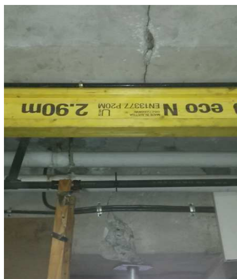
Photo 4.5.6 Exposed beam, with crack from slab visible propagating through beam
