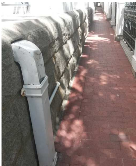
Photo 4.6.11: Position of Rainwater downpipe from roof correlates with position of severe corrosion of steel beams in basement.
