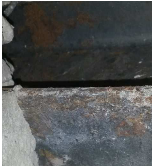
Photo 4.4.6: Bottom flange of beam that has almost no visible corrosion (+/- 6mm thick steel flange)
