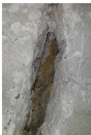
Photo 4.4.1: Exposed Steel beam edge with slight surface discoloration visible
