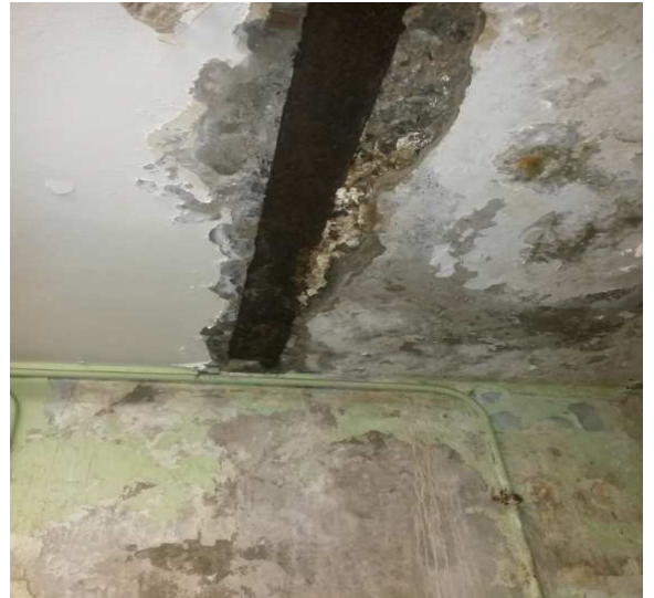
Photo 4.2.6: Another visibly corroded steel beam
