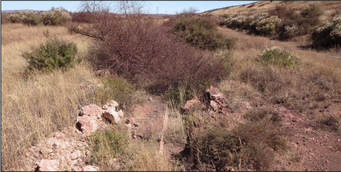
Figure 6: Existing solution trench overgrown with vegetation and filled with sediment
