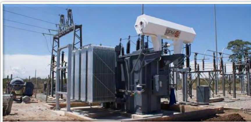
Substation with transformers at Sugarloaf Hill (Source: www.grocotts.co.za )
