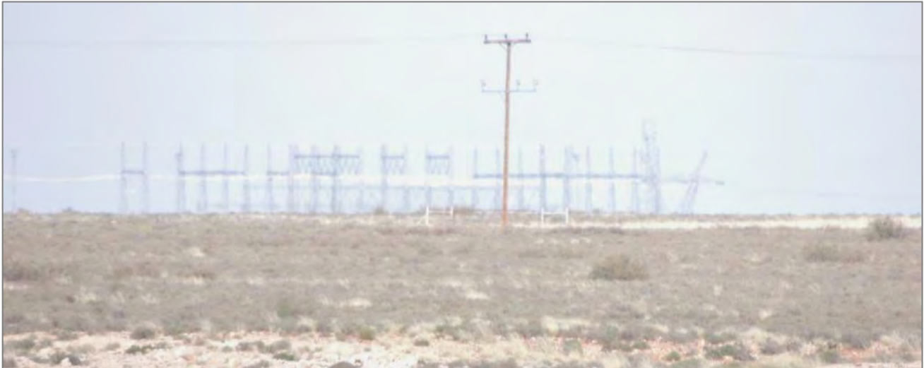
Figure 10: View of existing Cuprum substation
