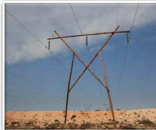
Example of an existing 142 kV transmission line (Source: VRMA)
