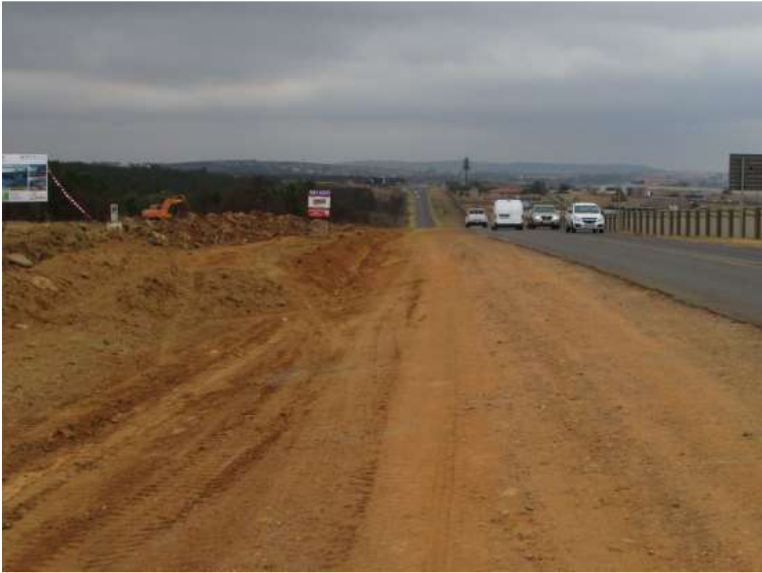
Figure 3: A section of the Eastern Link Sewer Line is located along the main Garstfontein Road.
