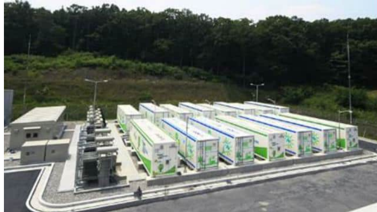
Figure 4: Example of a 15-container Lithium-Ion BESS installation
