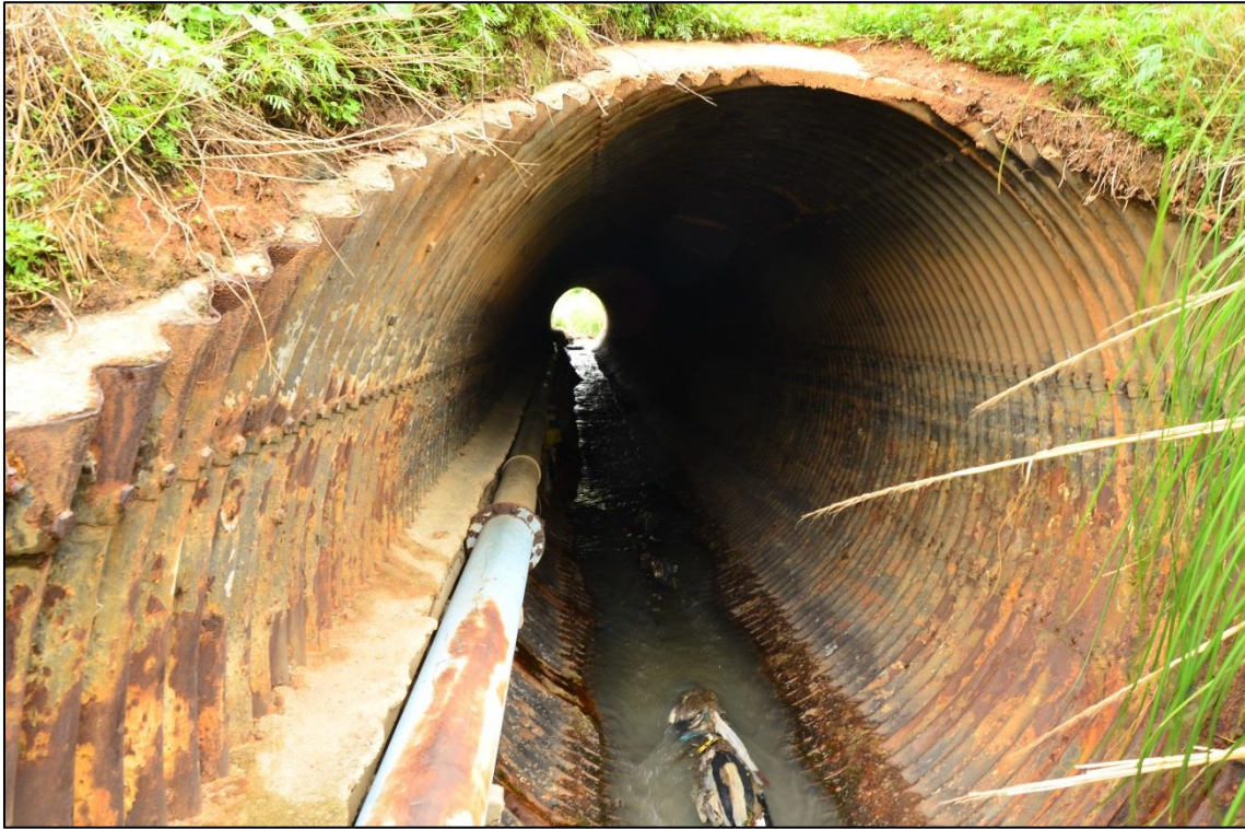
Figure 4-6: View of existing pipelines running under a road through a culvert. The proposed pipeline will also run along existing pipeline routes
