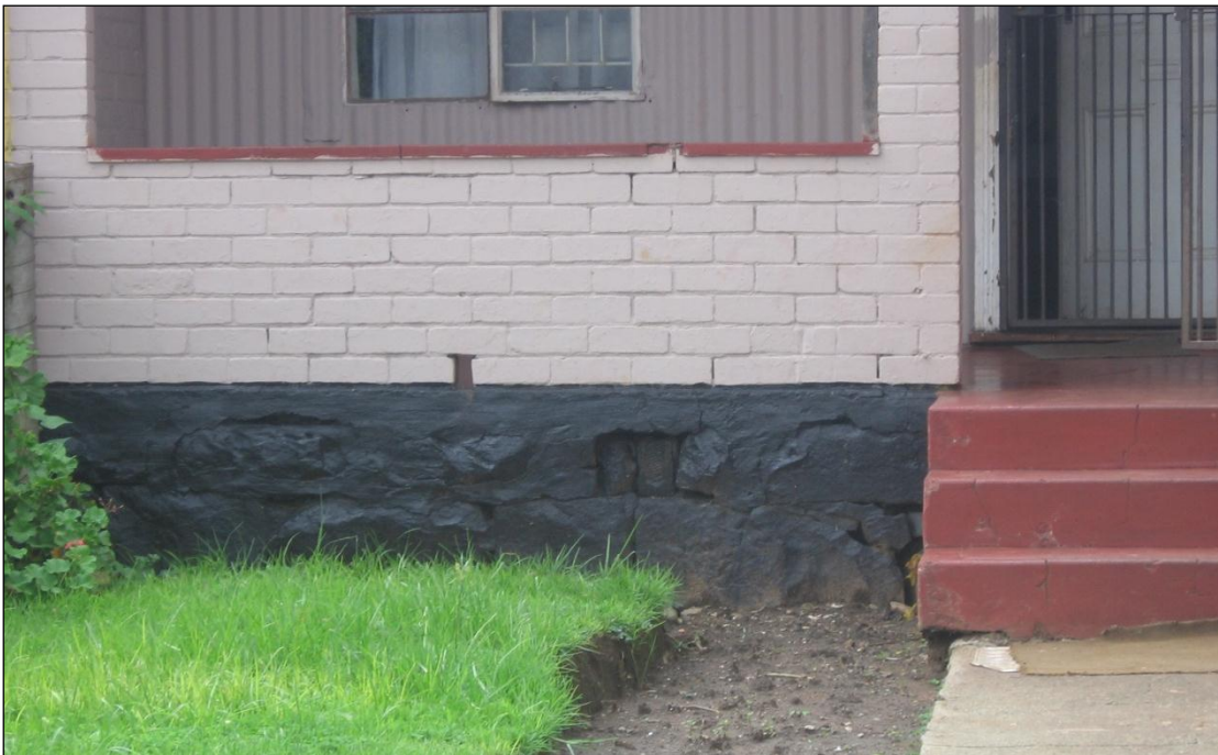
Figure 12: A section of the front elevation of another existing unit from the old married quarters. The original structure's corrugated iron sheeting and stone foundation can clearly be seen.
