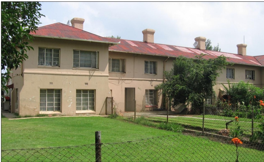
Figure 17: General view of the northern elevation of one of the units indicating the new steel frame windows that replaced the casement windows of Baker.
