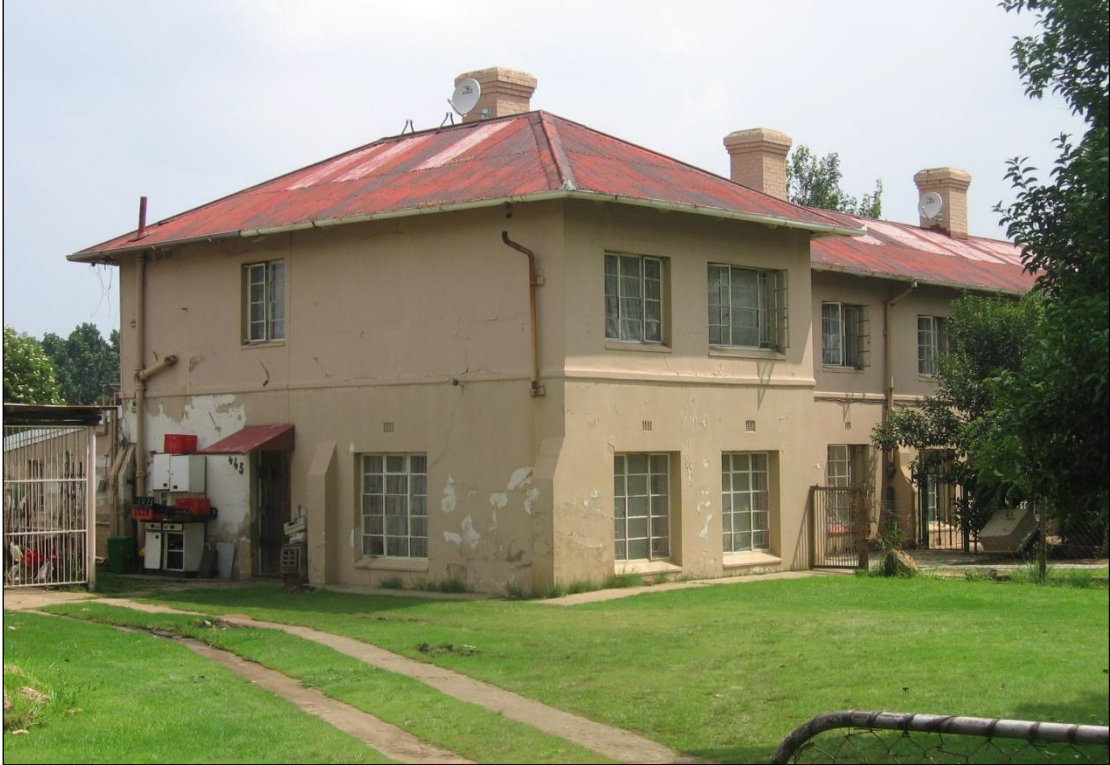
Figure 22: Corner elevation of one of the terrace buildings at ERPm with a slightly protruding pavilion and small buttressing element at its corner.
