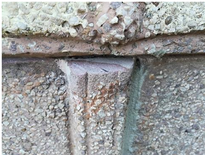
Figure 14: Patchwork on damaged area to obtain a uniform appearance of the panel element
