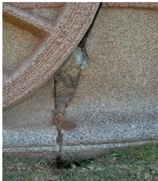
Figure 2: Example of previous repair work.
