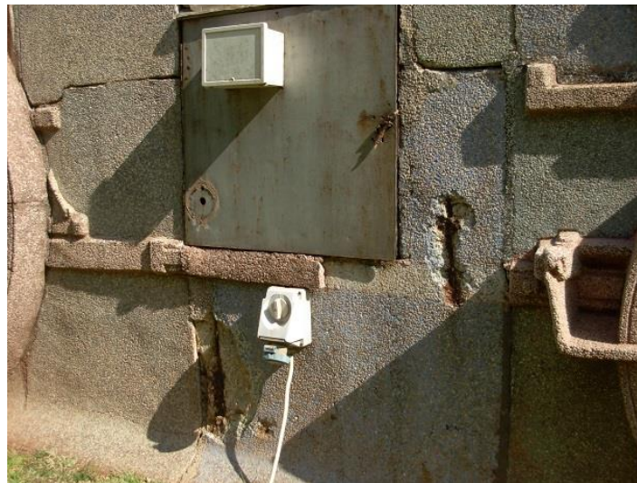
Figure 3: Example of current maintenance challenges – corroding metal reinforcement
