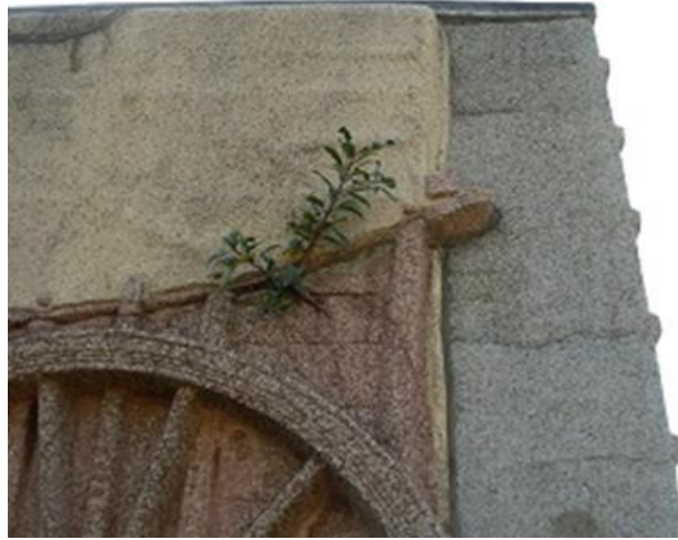
Figure 4: Example of current maintenance challenges – vegetation rooting in open joints
