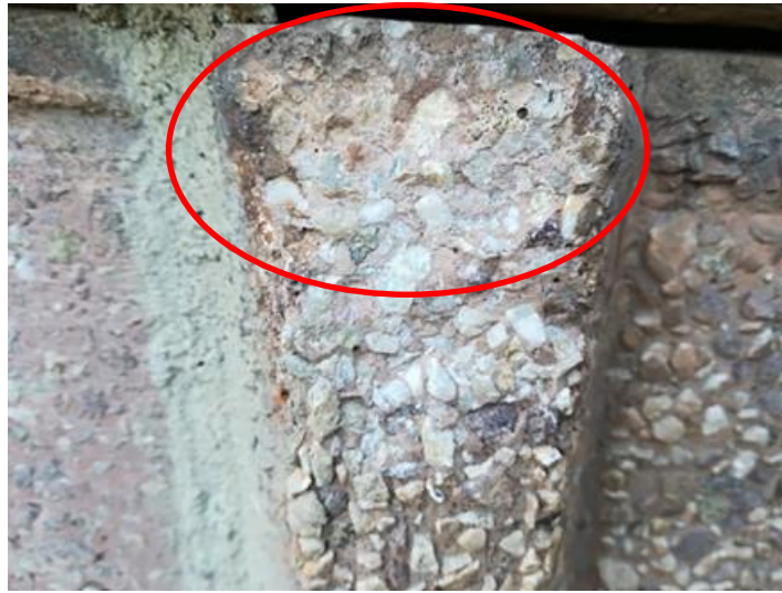
Figure 13: Example of superficial damage to a panel element.
