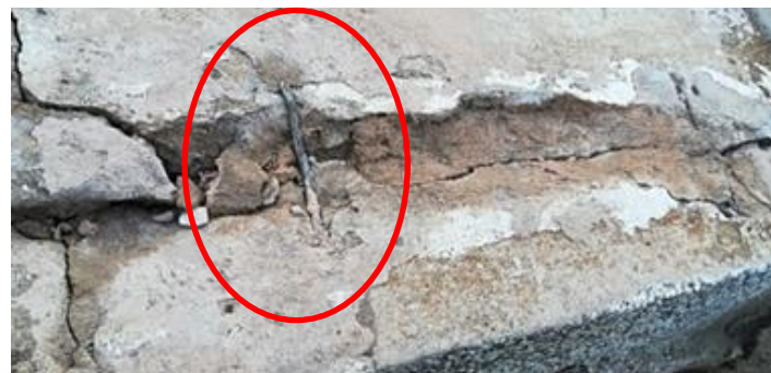
Figure 6: Example of copper staple inserted to join the panel to the concrete cast
