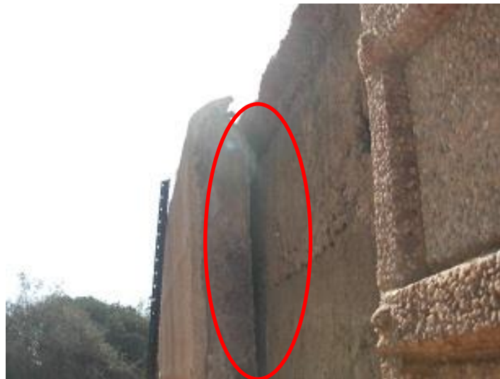
Figure 5: Example of original internal concrete cast behind a removed panel. Note the space between the panel and cast.
