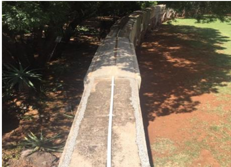
Figure 7: View of top part of wall after filling cavity and sealing of joints. White conduit contains electrical wiring.
