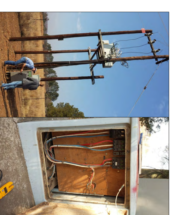
EXISTING POWER POLE & DB BOX
