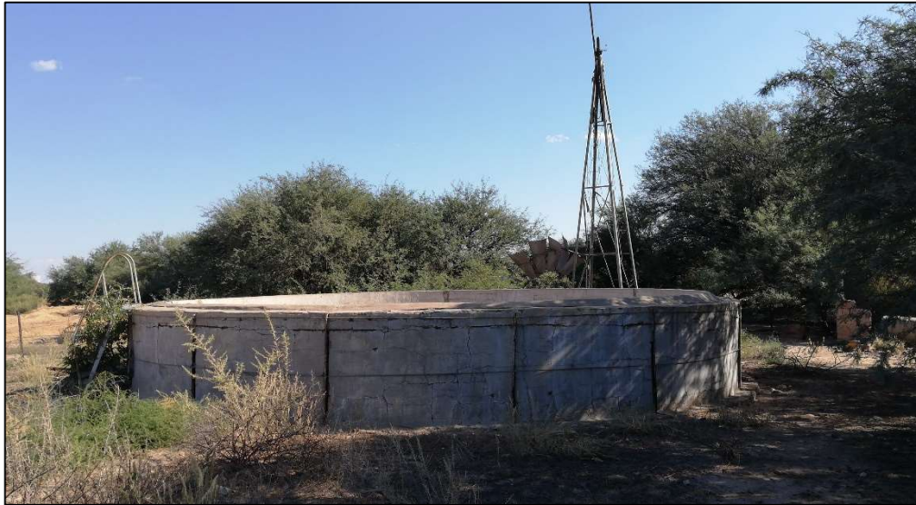
Figure 15: Windpump and reservoir at Site B01.
