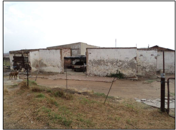
Figure 57: K06 – Dilapidated section.
