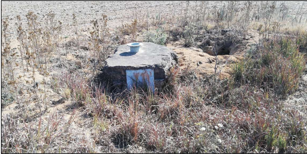
Figure 19: Irrigation system at Site K03.
