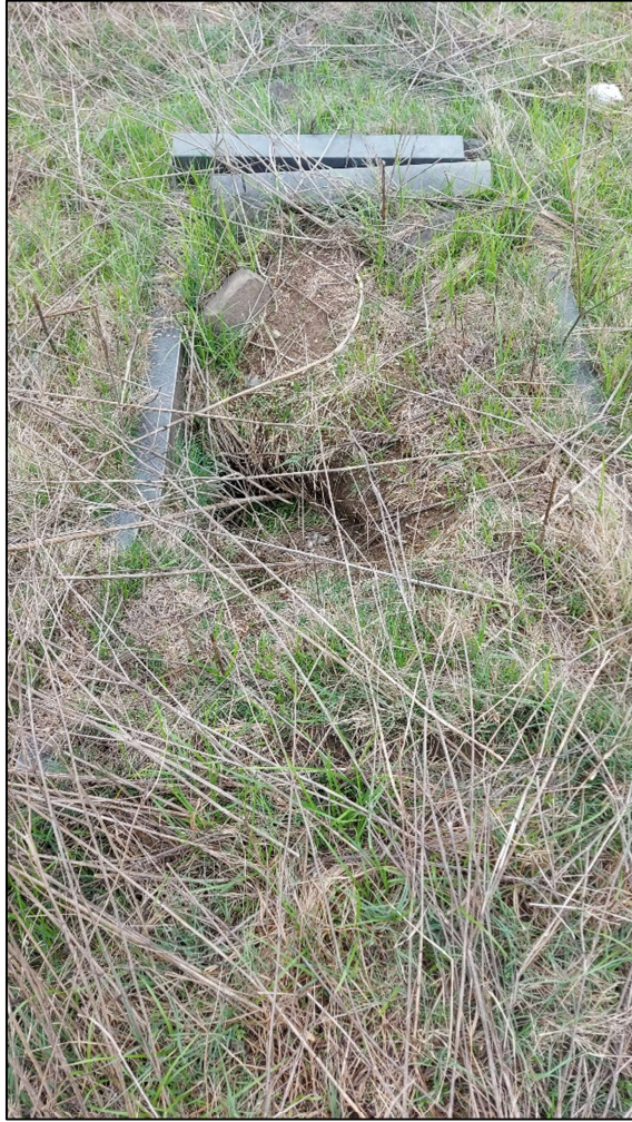
Figure 28: Dilapidated formal surface dressing at Cemetery F01.
