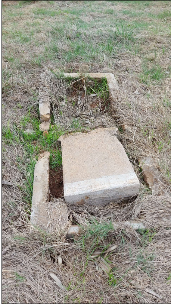
Figure 31: Dilapidated formal surface dressing of a grave at Cemetery F02.
