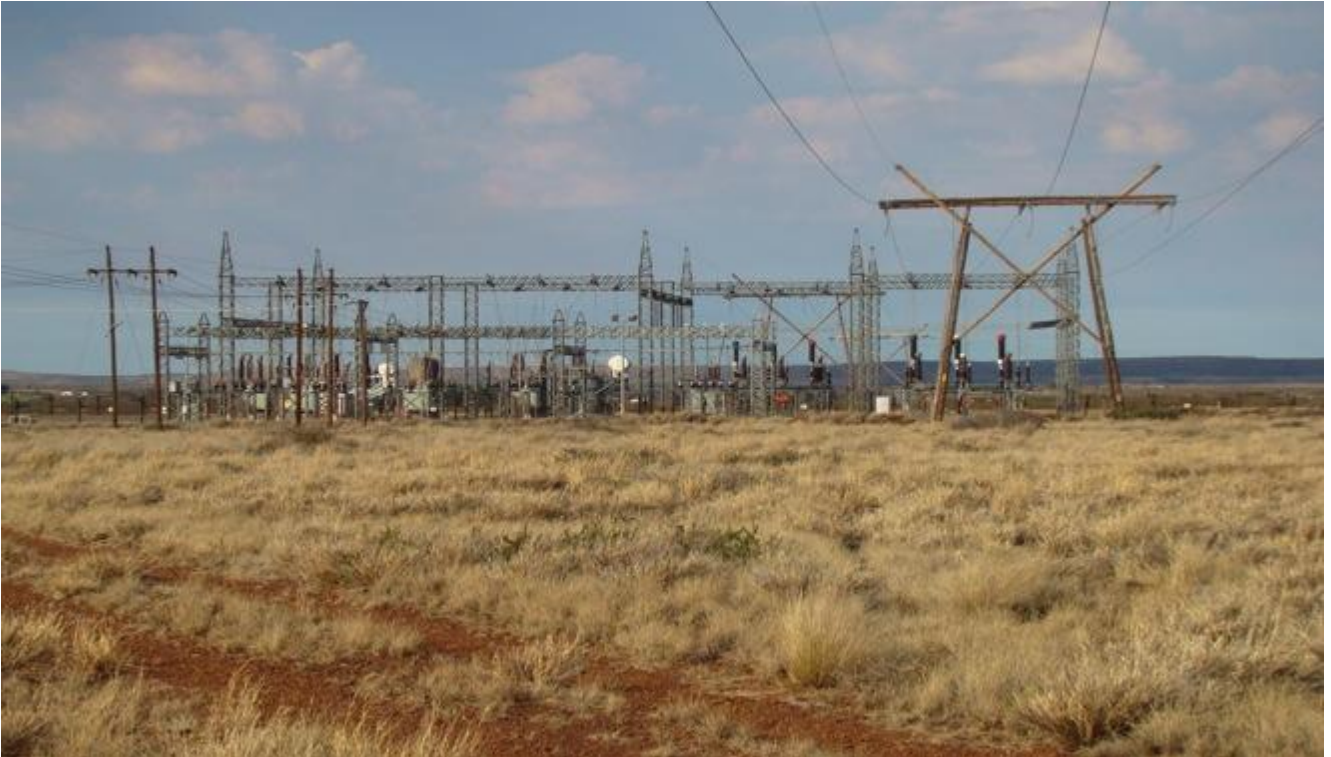
Plate 4: View of Eskom Substation situated on the periphery of the project area. This image also gives the typical cultural landscape within the project area. (Photograph © by Author 2012).
