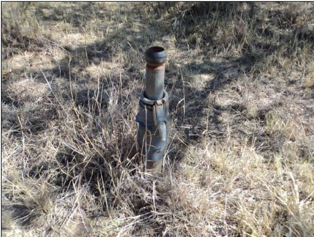
Figure 14: Irrigation system remains.
