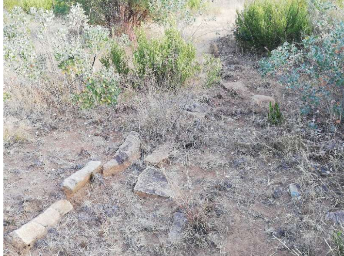
Figure 11: Example of dilapidated linear walling.
