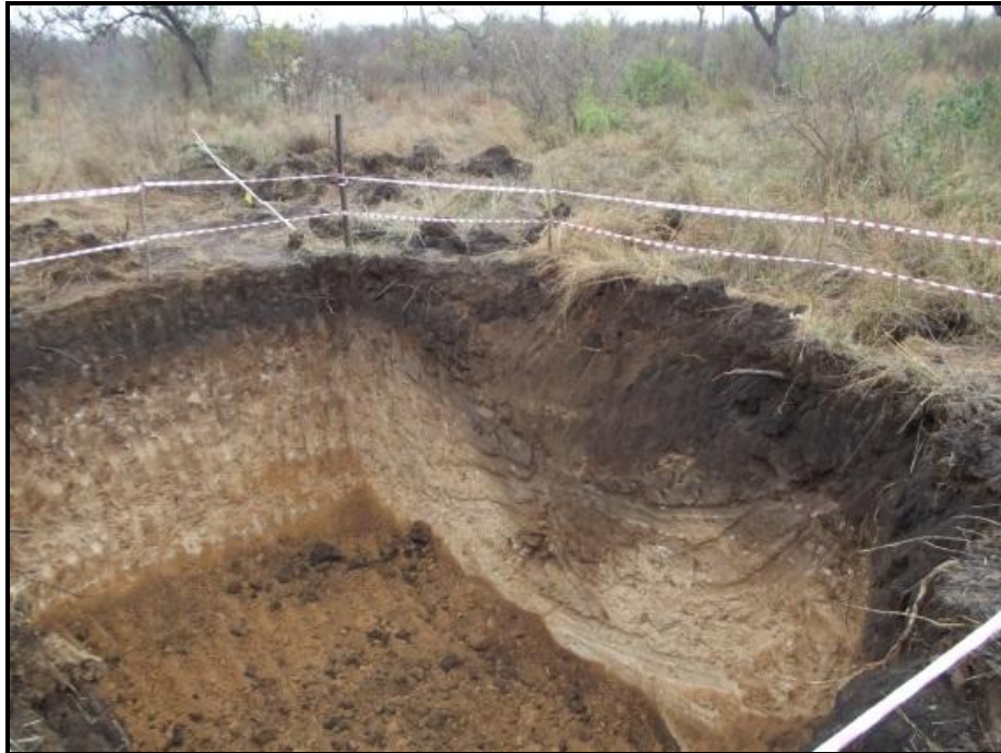
Fig. 6. A photo showing the profile of the hole where the septic tank will be placed.
