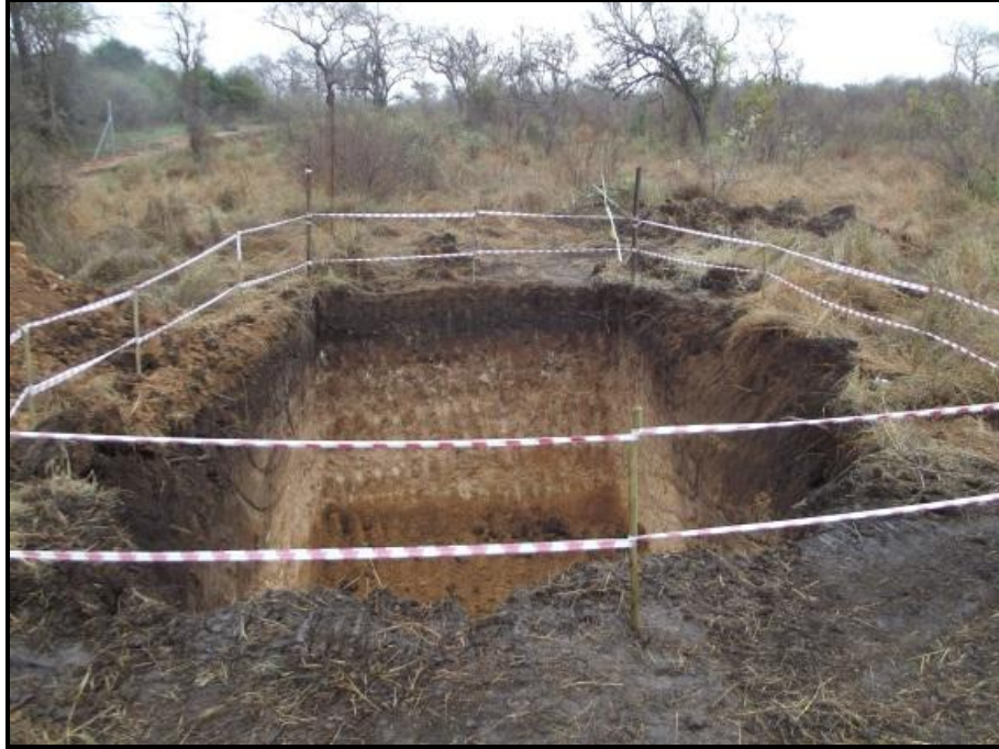
Fig. 5. A photo of the hole monitored where the septic tank will be placed.
