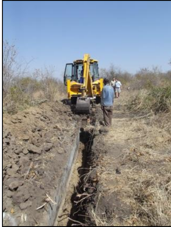
Fig. 5. An electric cable trench. Monitored on Aug 3, 2012. Photo taken In south-western direction.
