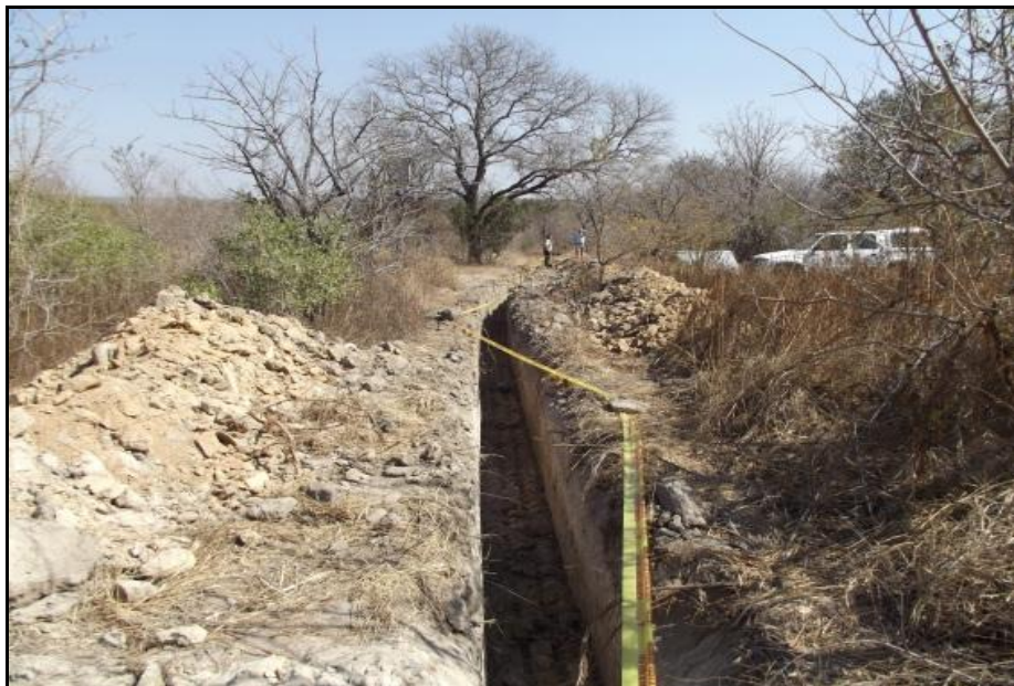
Fig. 4. The same sewage line as in fig. 3 where The line has turned east. Photo taken in western direction.
