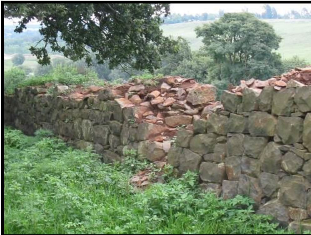
Figure 4. Stone walled livestock enclosure. This feature has been damaged in parts.
