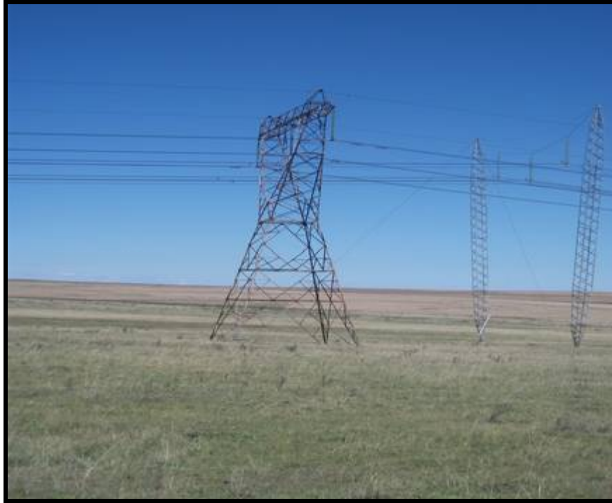
Power line crossing the site
