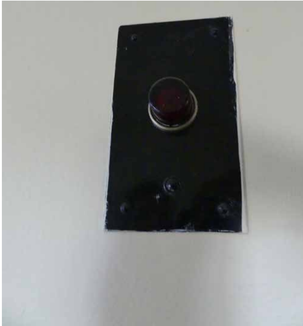
Alarm in ward on Third Floor- building 17.
