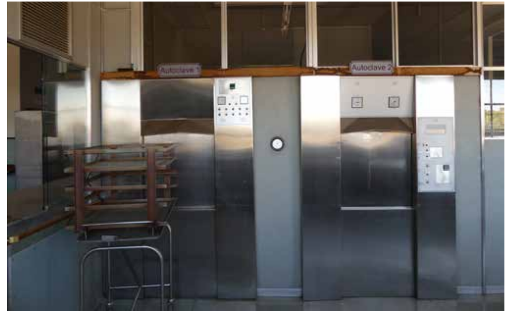
Sterilising unit on Second Floor - building 17.
