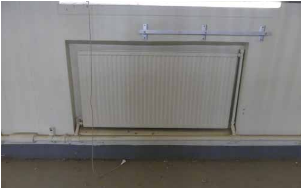
Heater in the wards (not original) - building 17.
