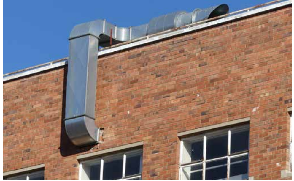
Air conditioners fitted to wards - building 17.
