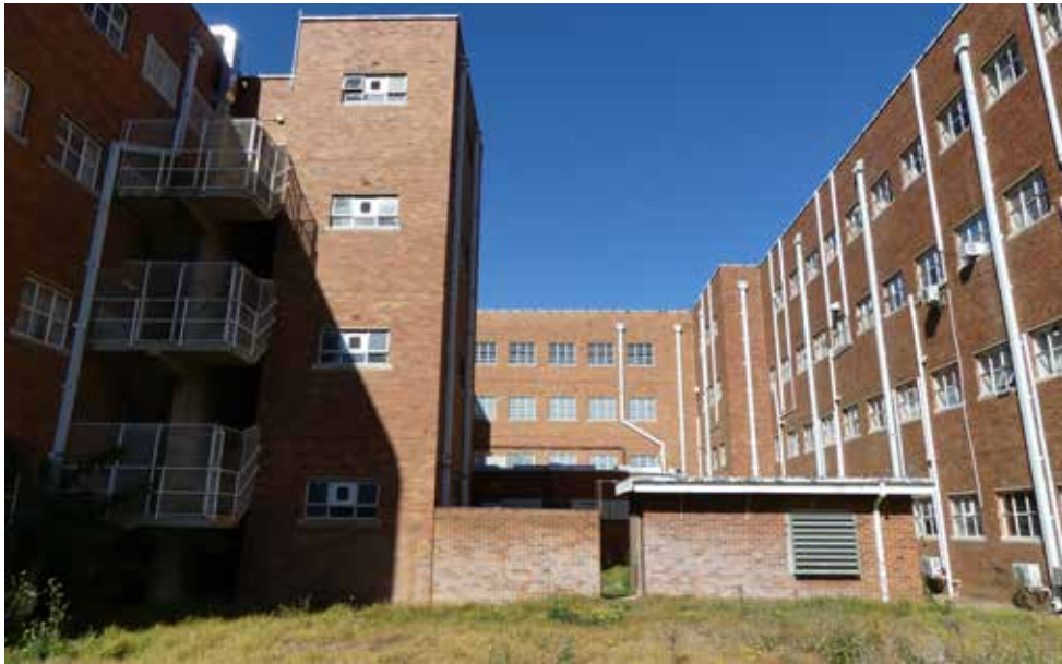
Fire escape to wards, extended toilet block and electrical room in front of ICU - building 17.
