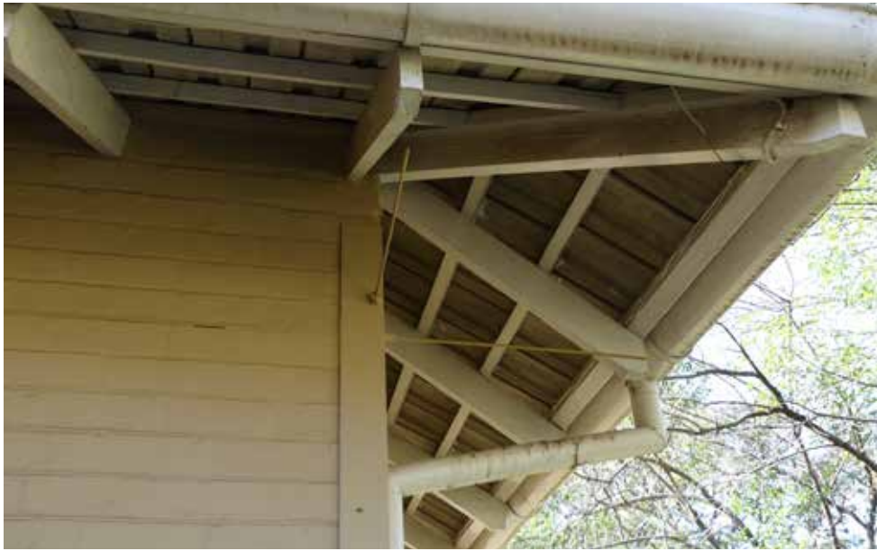
Underside of roof of building 4 - Doctor's House Type 5 - steel poles tying walls together.
