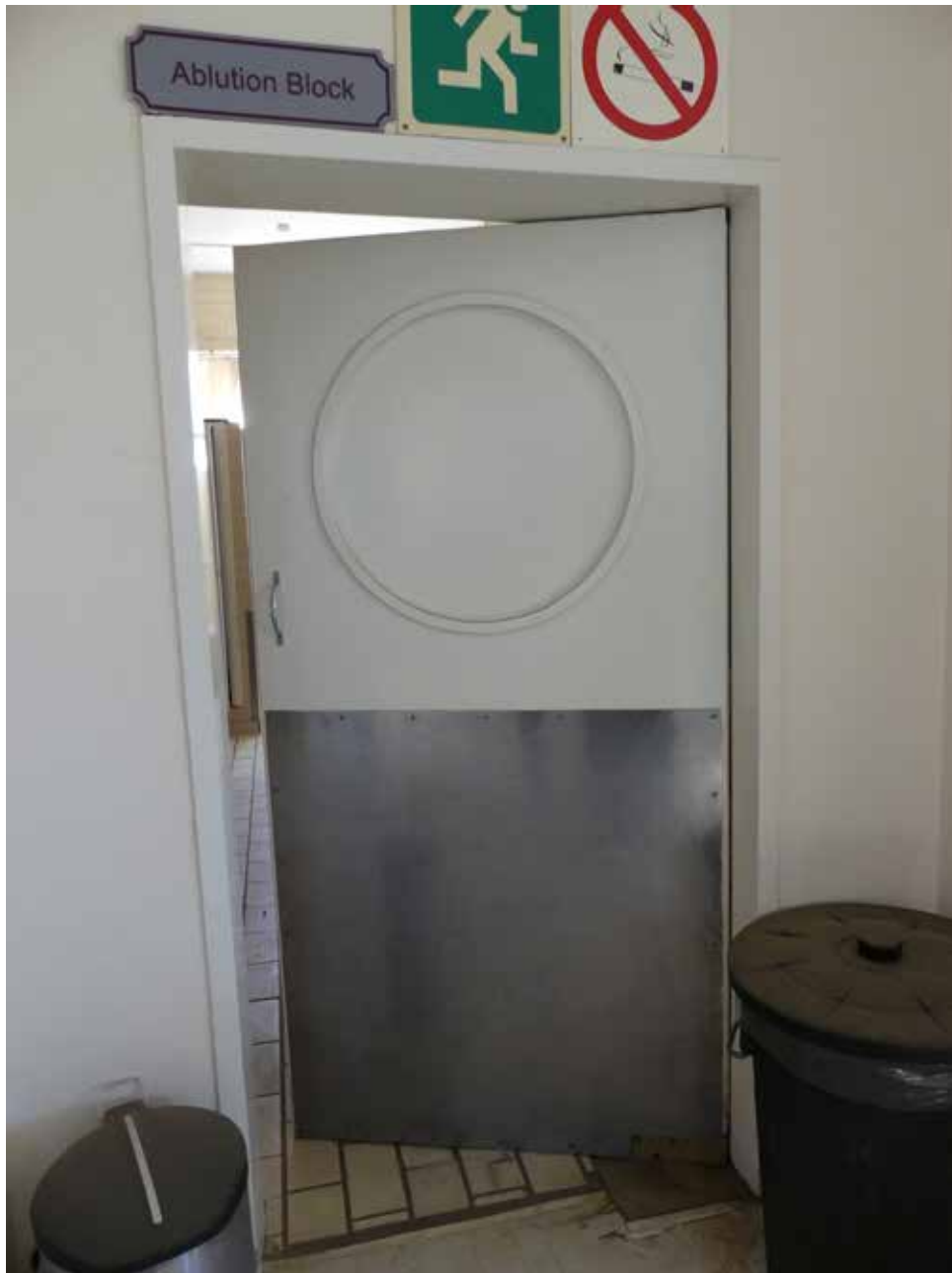
Original door to bathrooms off of the ward (modified with steel panel) - building 17.
