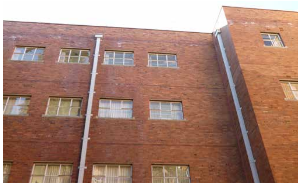
Original flat roof with pitched corrugated roof sheeting (behind the parapet) and down pipes - building 17.
