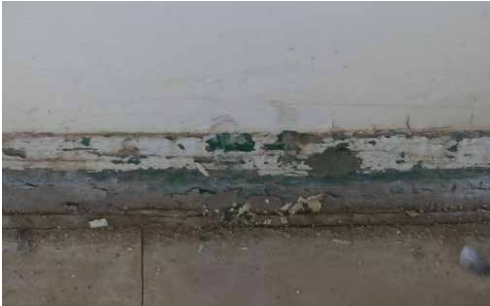
Detail of skirting on Third Floor - original skirting and flooring was green - building 17.
