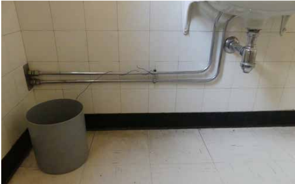
Original pipes and tiles in bathroom off of office in Admin (West) wing - building 17.
