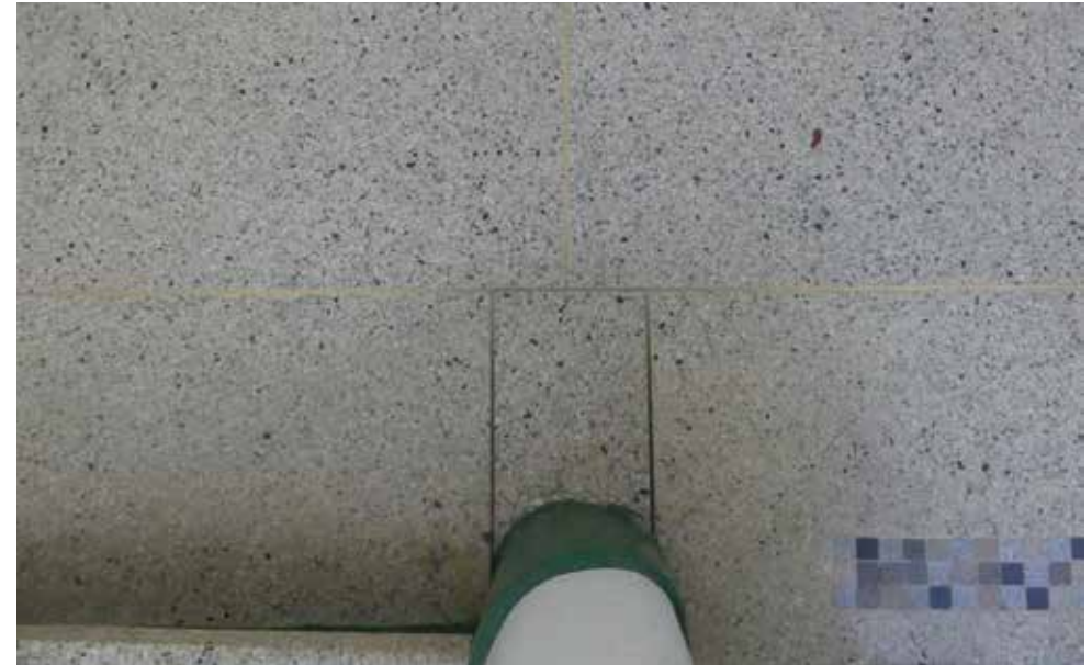
Original terrazzo and mosaic (with brass inserts) staircase to Admin (East) Block - building 17.
