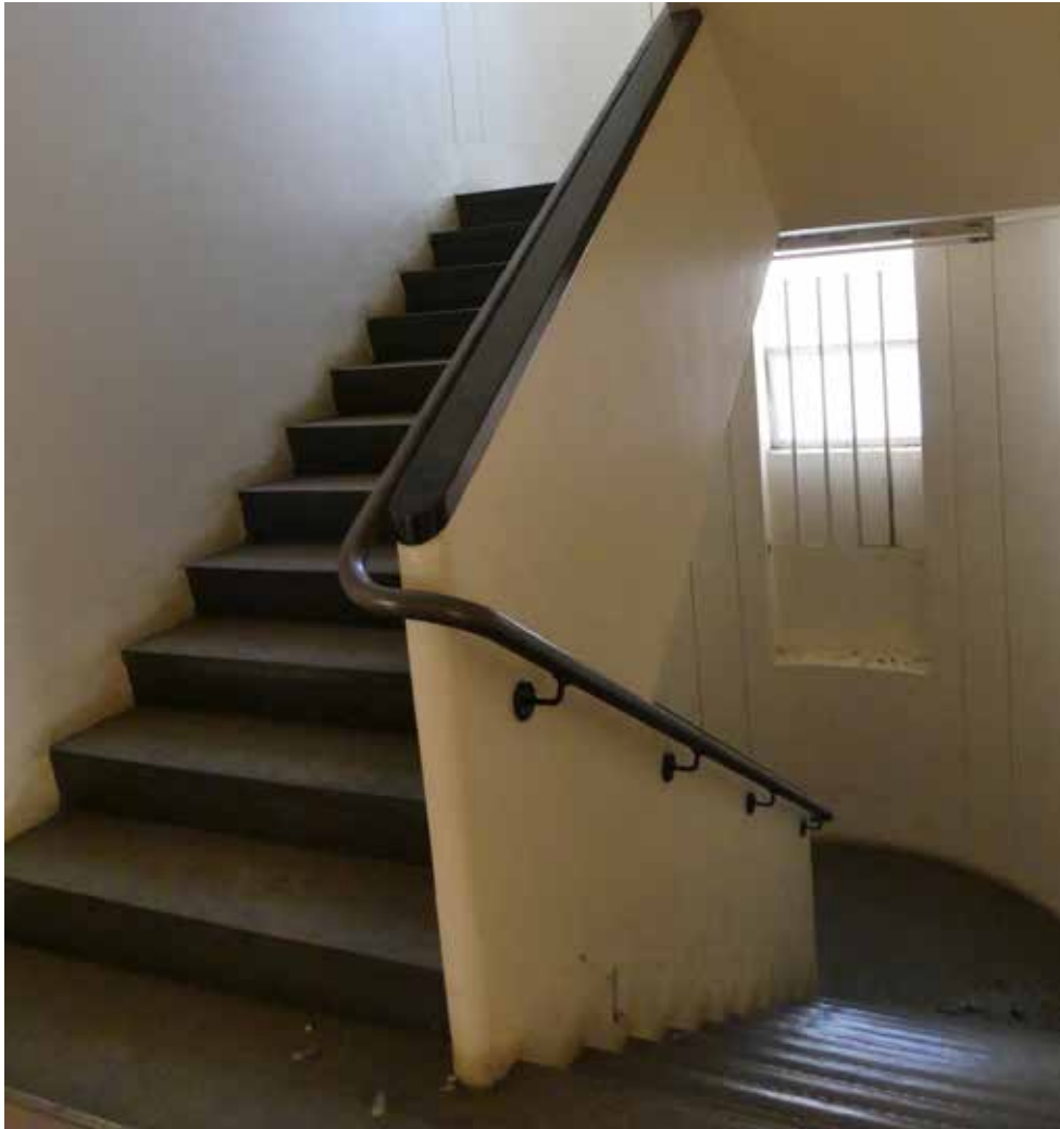
Original staircase (terrazzo and mosaic floor covered with vinyl) with original handrail - building 17.
