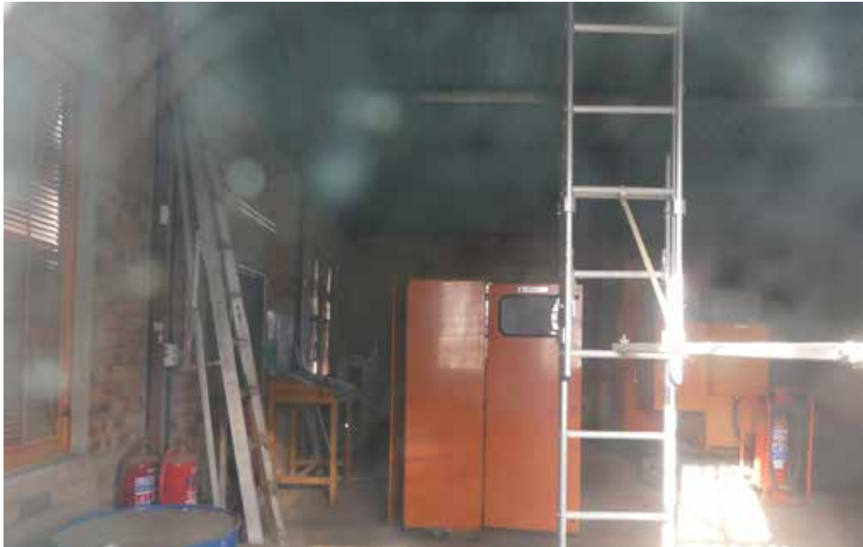
Interior of electrical room - building 34.
