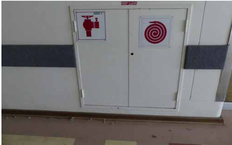
Original fire hose reel cupboard - building 17.
