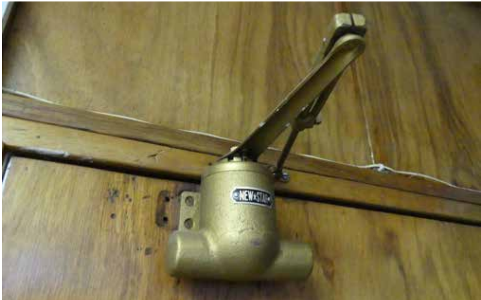
Door closer to Boardroom of the Admin Building - building 17.
