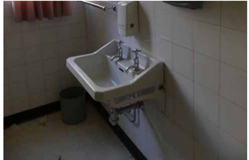
Original basin and tiles in bathroom off of office in Admin (West) wing - building 17.
