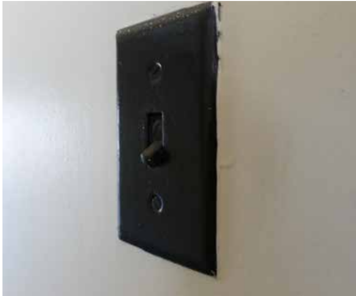
Original light switch - building 17.
