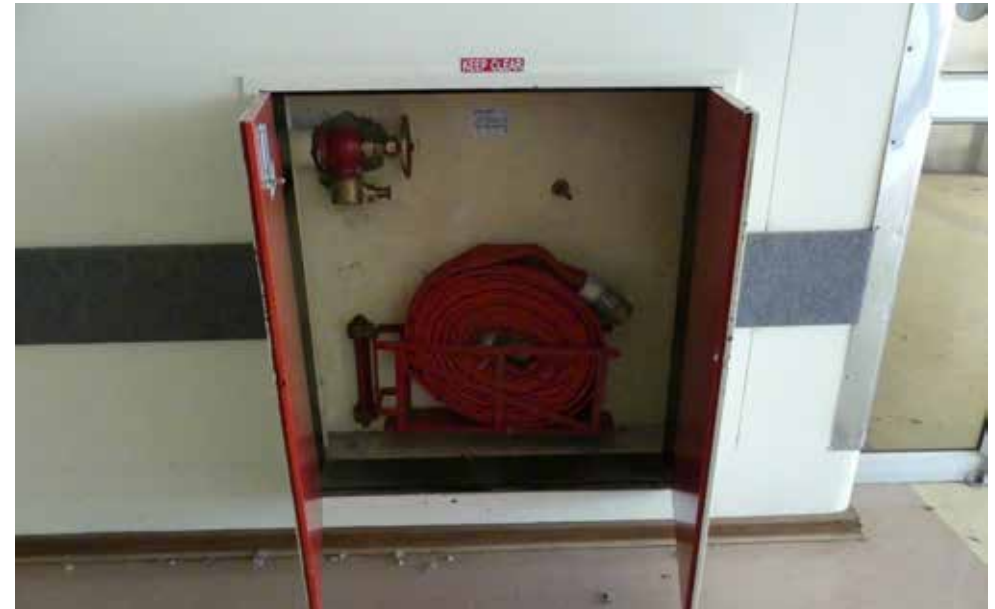
Original fire hose reel cupboard - building 17.
