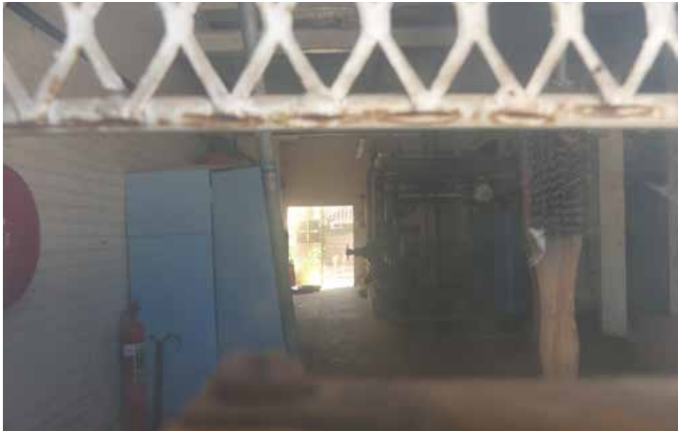
Interior of Boiler Room - building 32.
