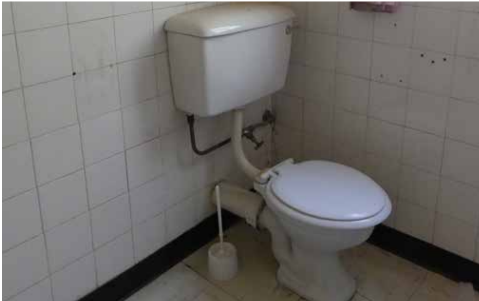
Original WC and tiles in bathroom off of office in Admin (West) wing - building 17.
