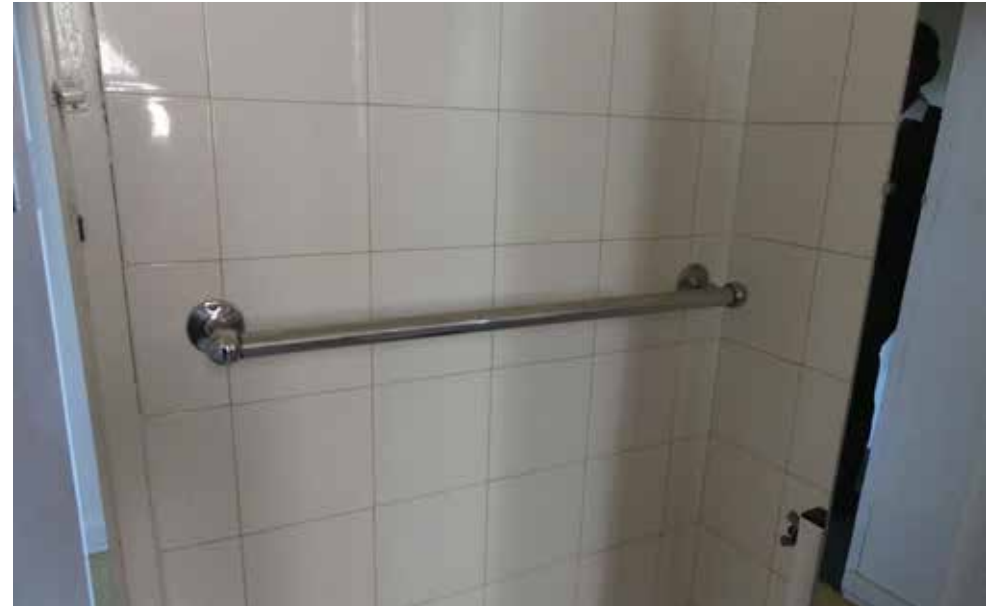
Original towel rail and tiles in bathroom off of office in Admin (West) wing - building 17.
