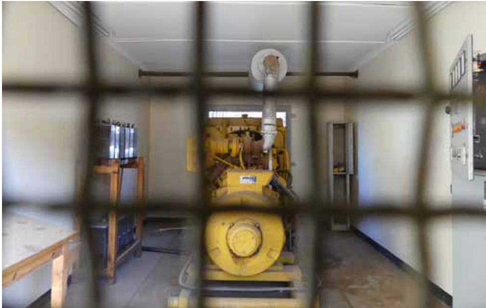
Interior of Boiler Room - building 32.
