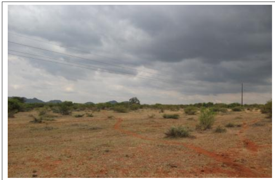
Figure 10- The 132kV power line between Dithabaneng and the proposed Dwaalkop Substation runs across an open plain to the north-western corner of the village of Makurung (above).
