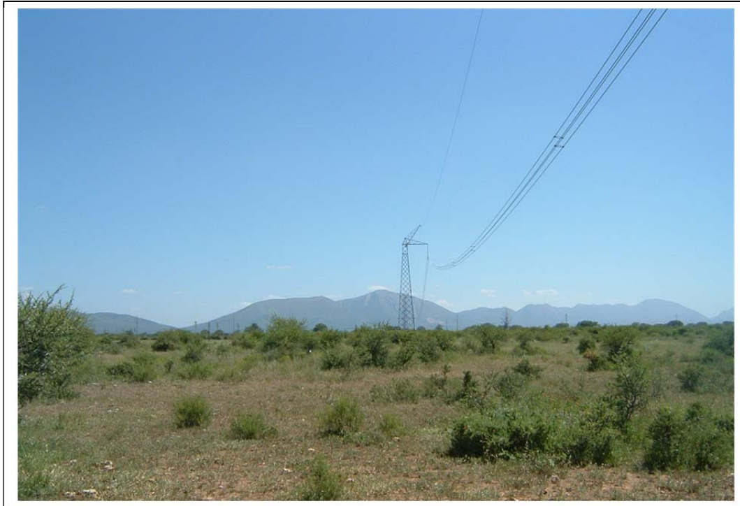
Figure 6- Long stretches of the preferred and both the alternatives routes for the 132kv Gompies to DWAF02 Substations power lines follow the existing Caborah Bassa power line where no heritage resources were observed. This corridor has been disturbed as a result of earlier construction activities (above).
