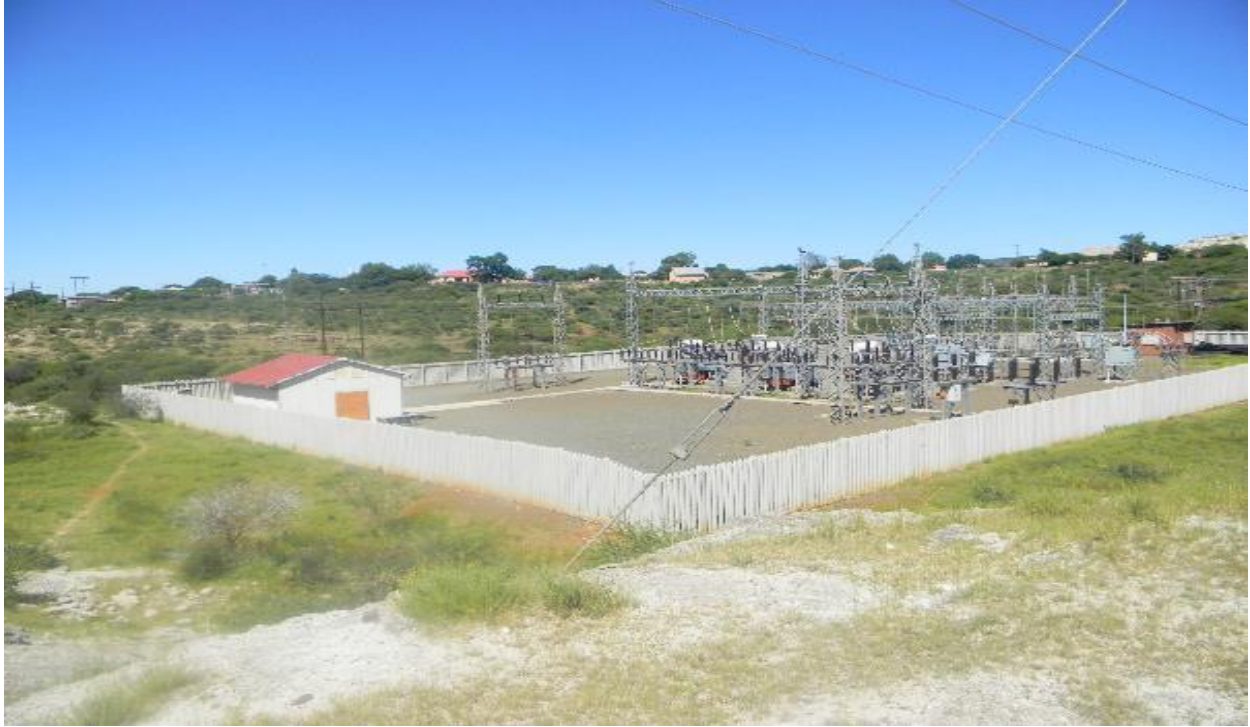
Figure 5: view of Norlim Substation where the proposed power lines will T-off from
