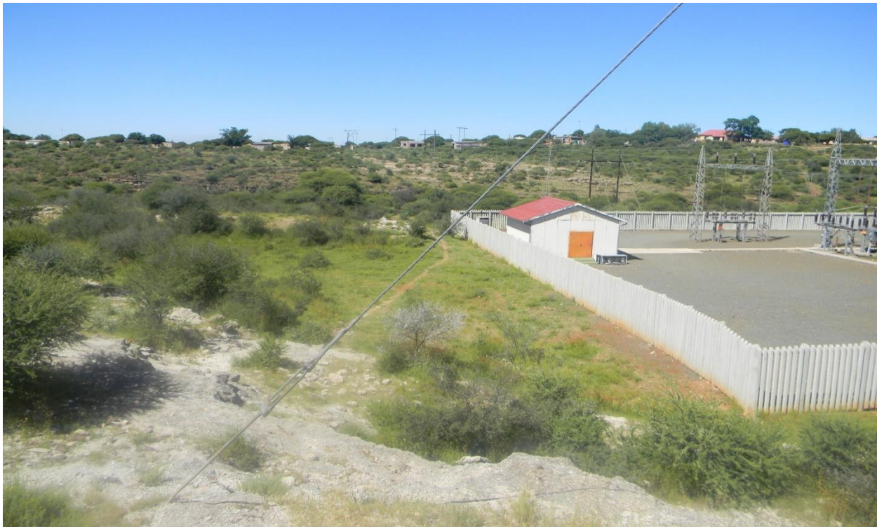
Figure 6: View of Norlim Substation and power line route running along existing power line servitude
