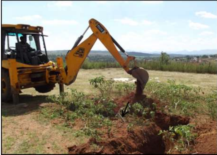
Figure 9. Trenches were opened around the peg which marked the spot where the remains were found (see arrow).
