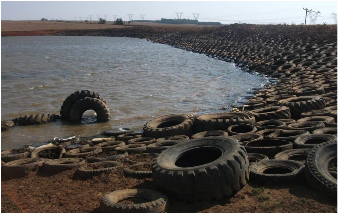
Figure 3: Dam wall with layer of tyres to prevent erosion of the wall
