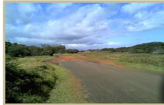
EXISTING ROAD DUE FOR REALIGNMENT- DAMAGE DUE TO INUNDATION
