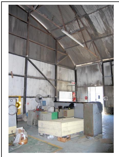
Fig. 18 North-west corner, note the lack of cross bracing on the north wall. The same is visible in Fig 14.
