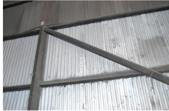
Fig. 14 A column with a diagonal timber brace. There was no obvious means of mechanical connection between the timbers.
