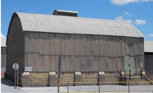
Fig. 8 View of the north-facing façade with inside the air vent on the top of the roof.
