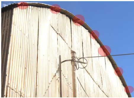
Fig. 15. Irregular cutting of the roof sections support the hypothesis that the structure was cut and shortened
