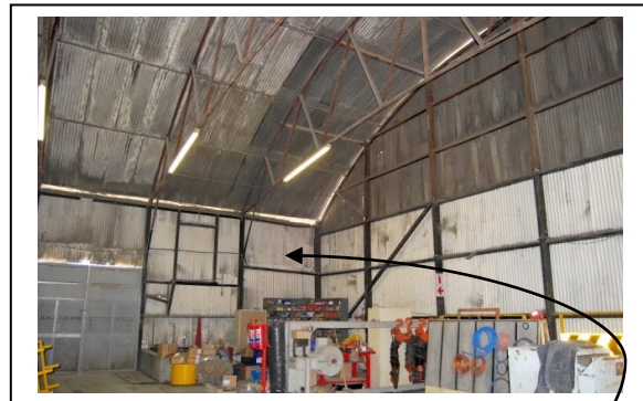
Fig. 23 South-west corner which ties in with Fig 16. Note the lack of cross bracing
