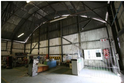
Fig. 10 View of the clear-span structure of the building looking towards the West gable.
