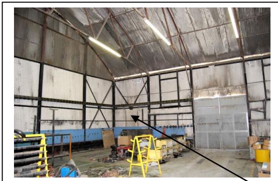
Fig. 22 South-east corner with double door. Note the missing lower cross braces.
