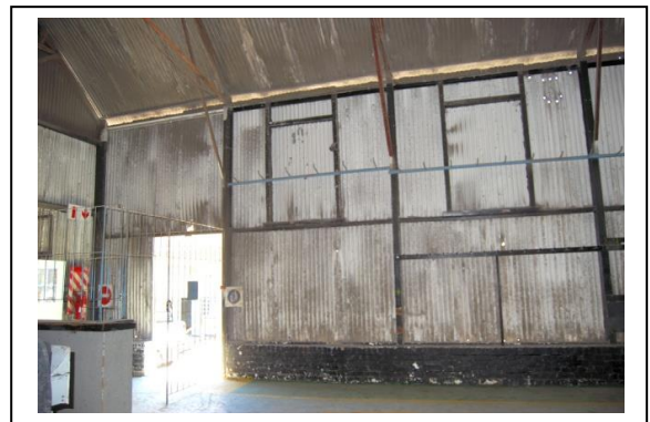
Fig. 19 North wall by doorway. The rectangles on the wall are timber frames of earlier windows.
