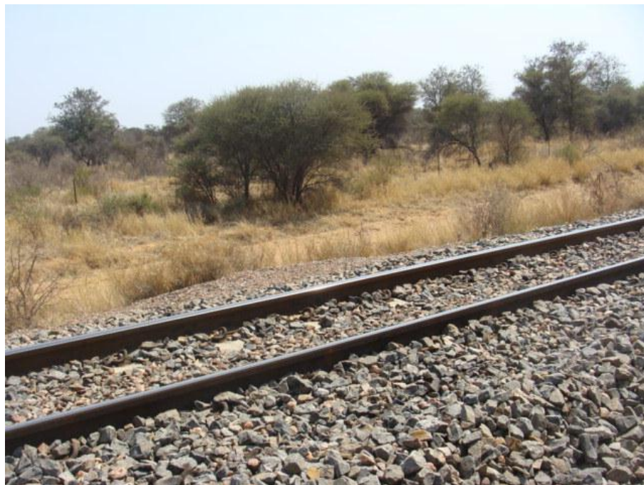
Figure 10: Existing railway track inside of the surveyed area on the farm Hanglip.
