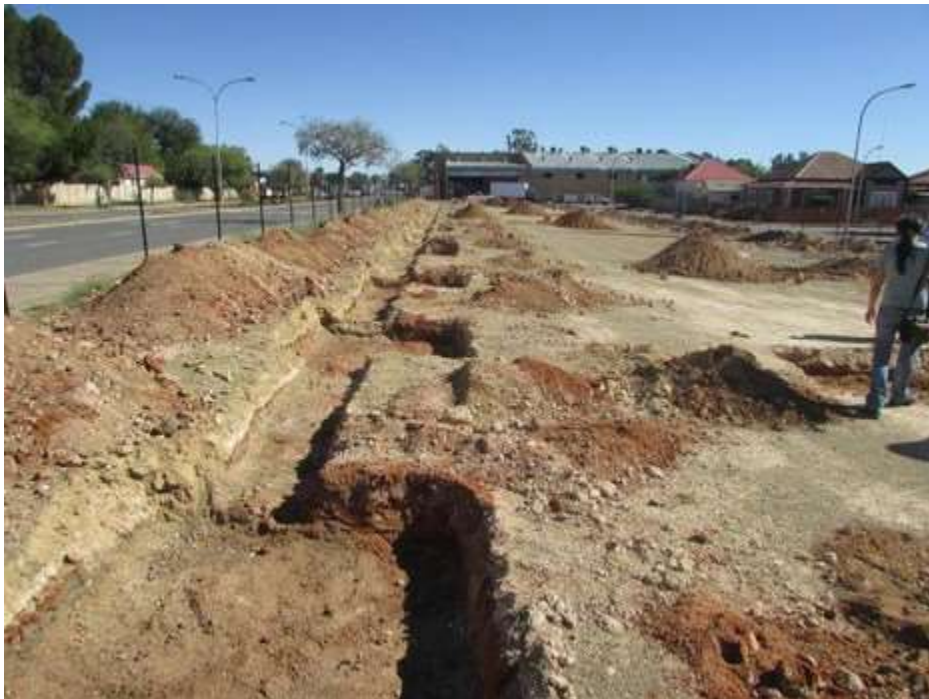
Figure 5: A closer view of the foundation trenches taken down Quinn Street towards Lawrence Street.
