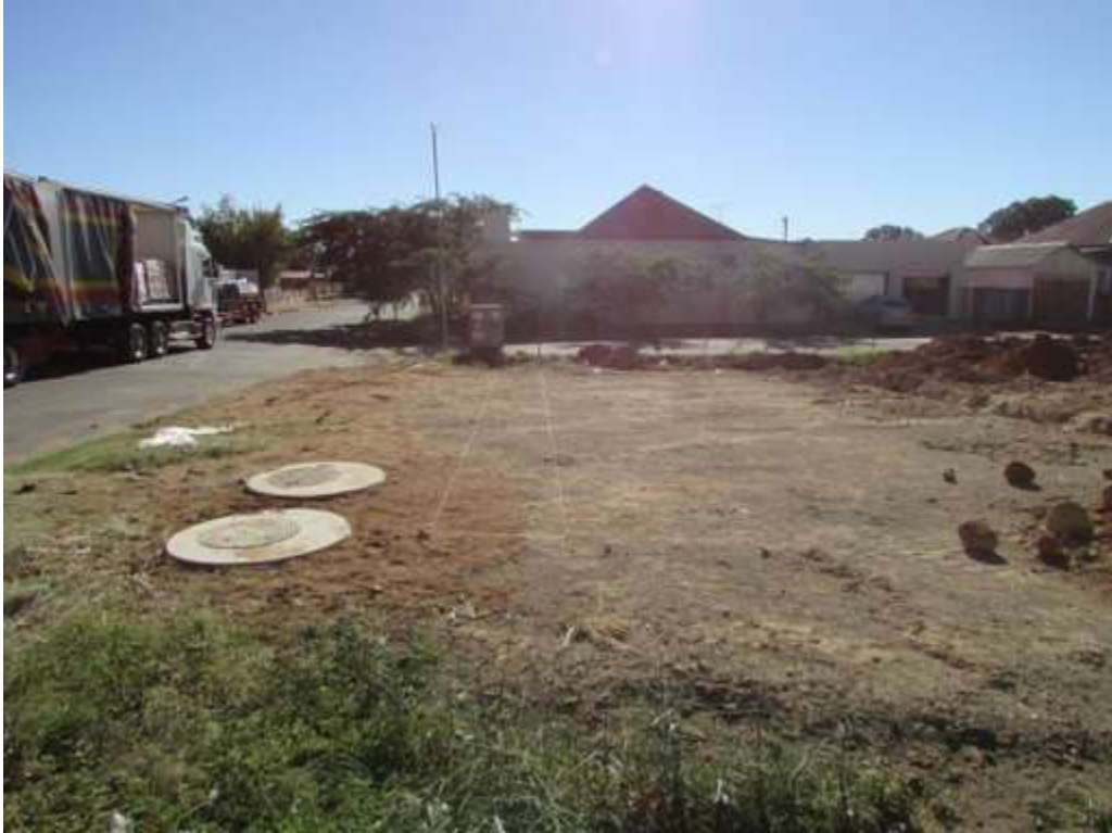
Figure 9: Test Trench 1 prior to excavation. The man-holes show the approximate Neotel Line connection.
