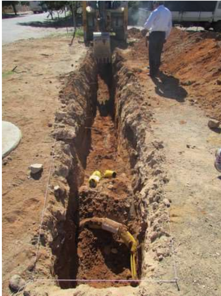
Figure 10: TT1 being excavated. A section of the Neotel Line connection was exposed.
