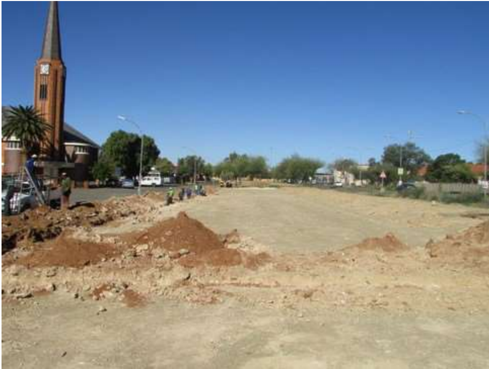
Figure 4: The development area taken from Lawrence Street towards the east showing the foundations test trenches being dug.
