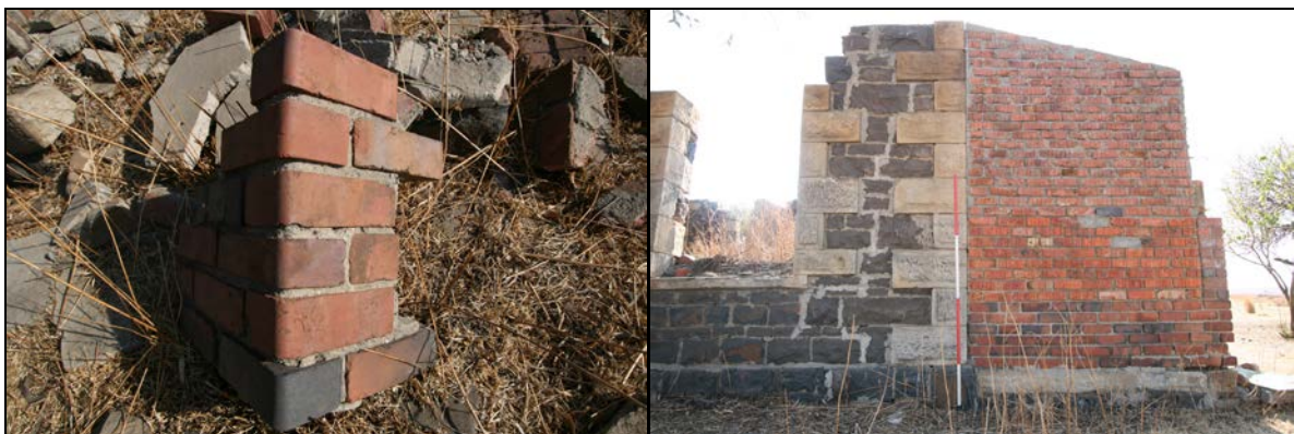
Figure 26: The rounded edges of clay bricks used for the pillars and the addition of an outside toilet on the verandah (Phase 3B type clay bricks)
