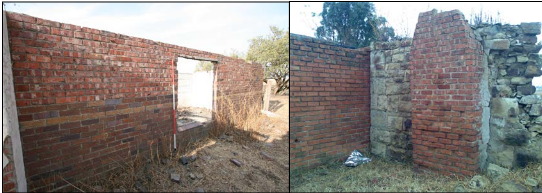
Figure 27: Outside wall of the main Phase 3B room; the external brick chimney added to the west-facing stone wall of Phase 2A/2B
