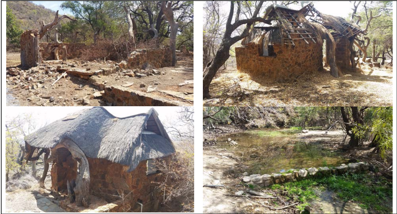
Figure 8: Dilapidated structures at the hunting camp near Lotteringskop (also note perennial spring)
