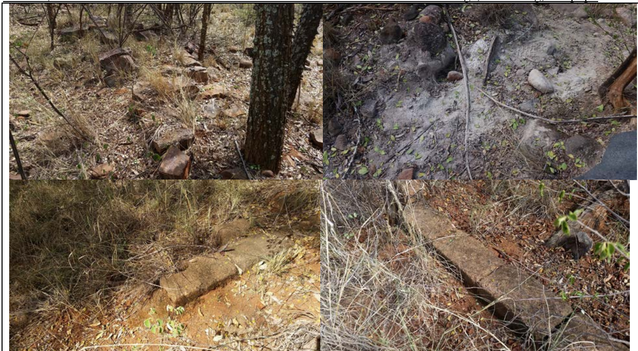
Figure 20: The foundation of the historical farm complex and ashy midden to the rear of the yard
