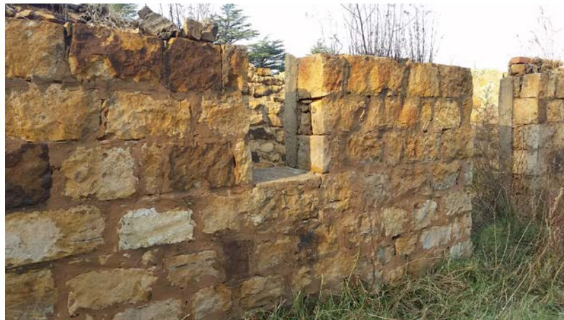
Figure 42: All the fittings of the main structure have been removed
