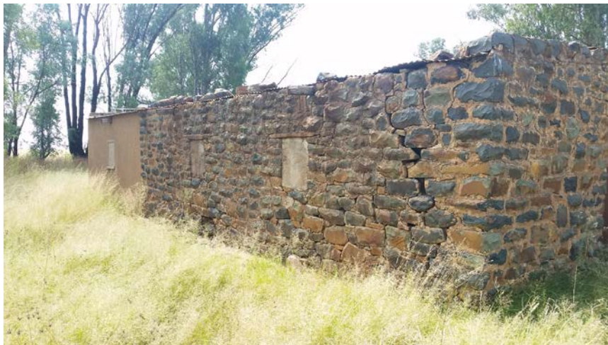
Figure 33: The farmhouse is structurally unsound
