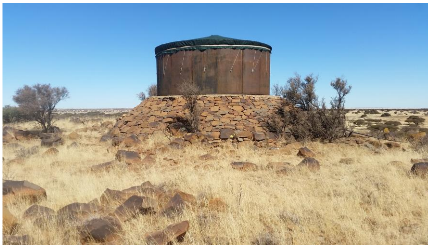
Figure 34: Water reservoir consisting of iron plates revited together, standing on a stone platform
