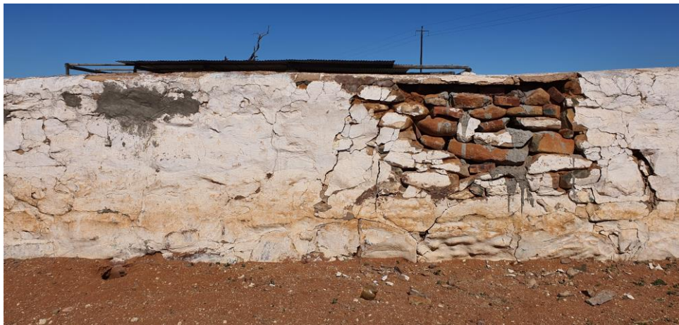
Figure 40: Front section indicating the unstable section of the walling
