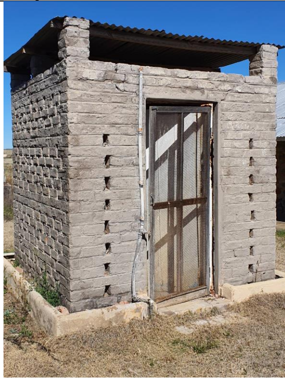
Figure 44: A general view of the cooler situated adjacent to the main house
