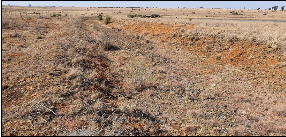
Figure 20: General view of the central section of the survey footprint (old railway line, track removed)
