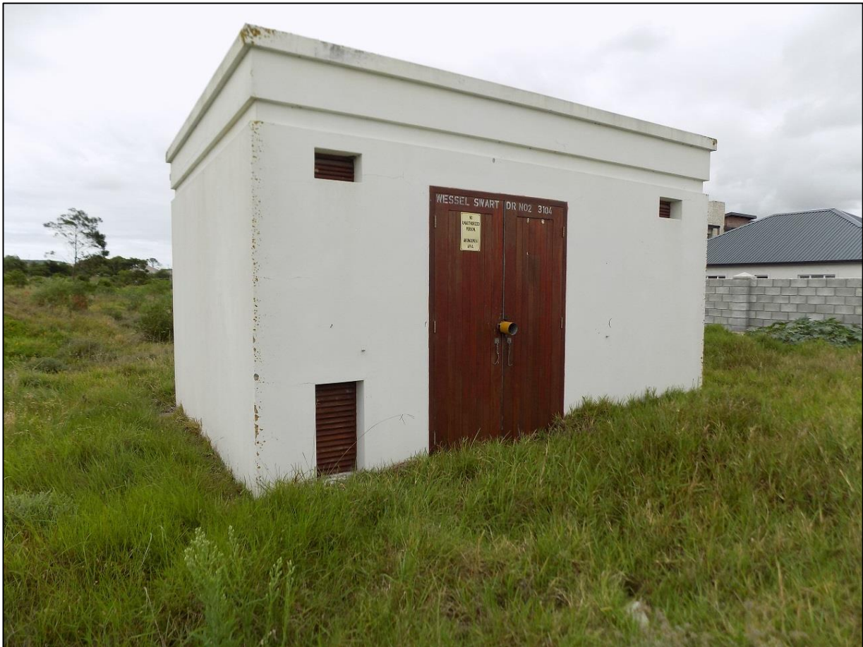
Figure 1. General view of the electrical transformer station that is located within the proposed development area on on Erf 4033 in Fairview, Gqeberha (Port Elizabeth), Nelson Mandela Bay Municipality, Eastern Cape Province.
