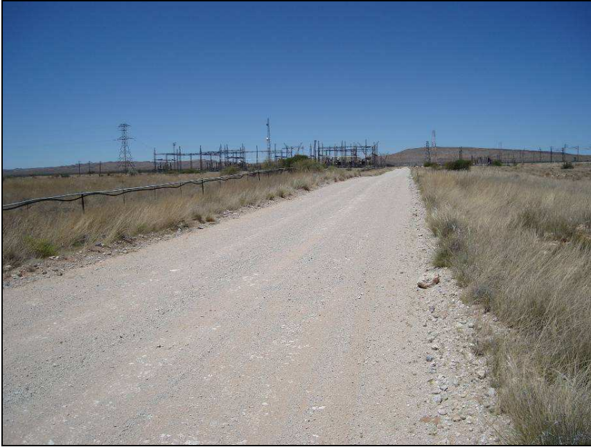
Fig.1 Garona Sub-Station near Groblershoop (Point 1 Map 10).
