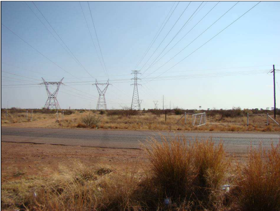
Fig.12 Pylon K4 outside Kathu.
