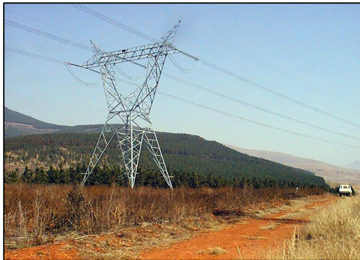
Figure 3: Self-Supporting Strain Tower
