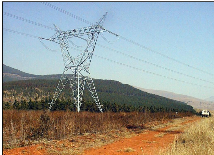
Figure 3: Self-Supporting Strain Tower
