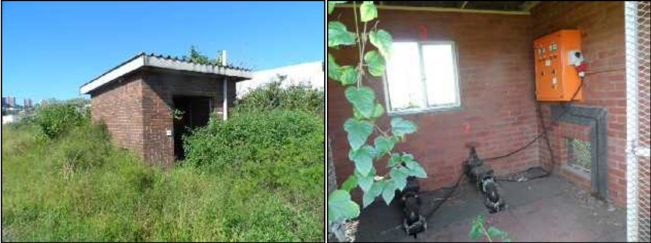
Figure 20- Pump house. Note the water pipes and the electric power box
