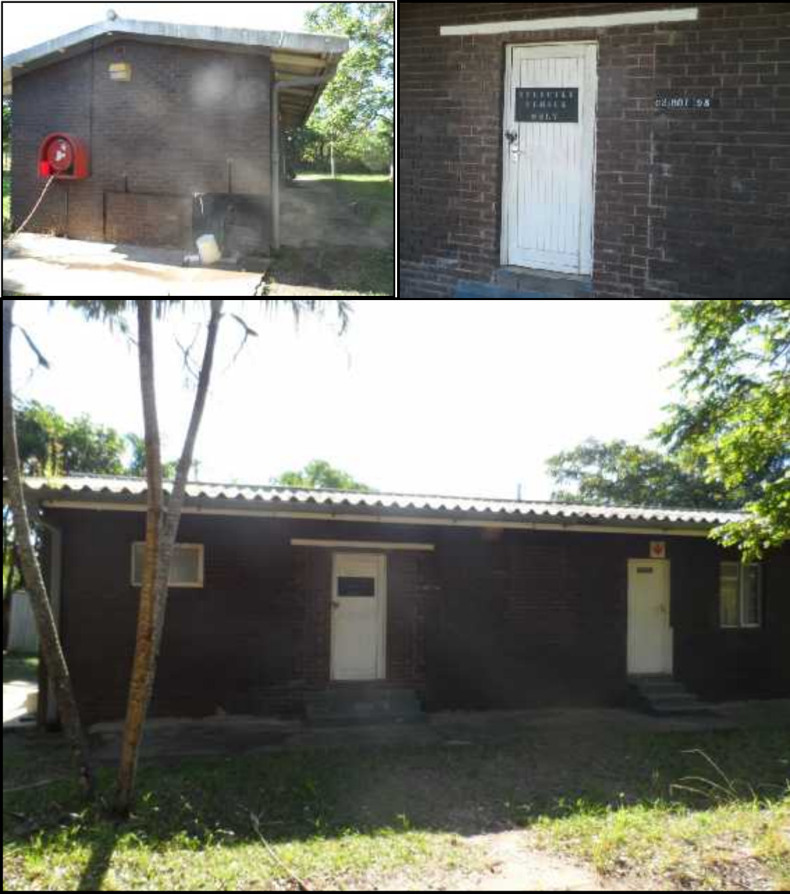
Figure 17- Female ablution and changing rooms. Note the alterations on the structures to seal off windows and to put new doors. The facilities are also clearly gendered (strictly female-upper right)
