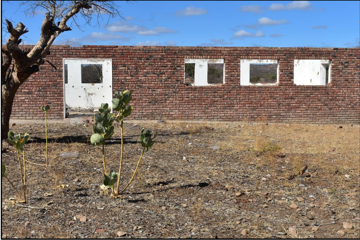
Figure 8: Two room dilapidated structure.
