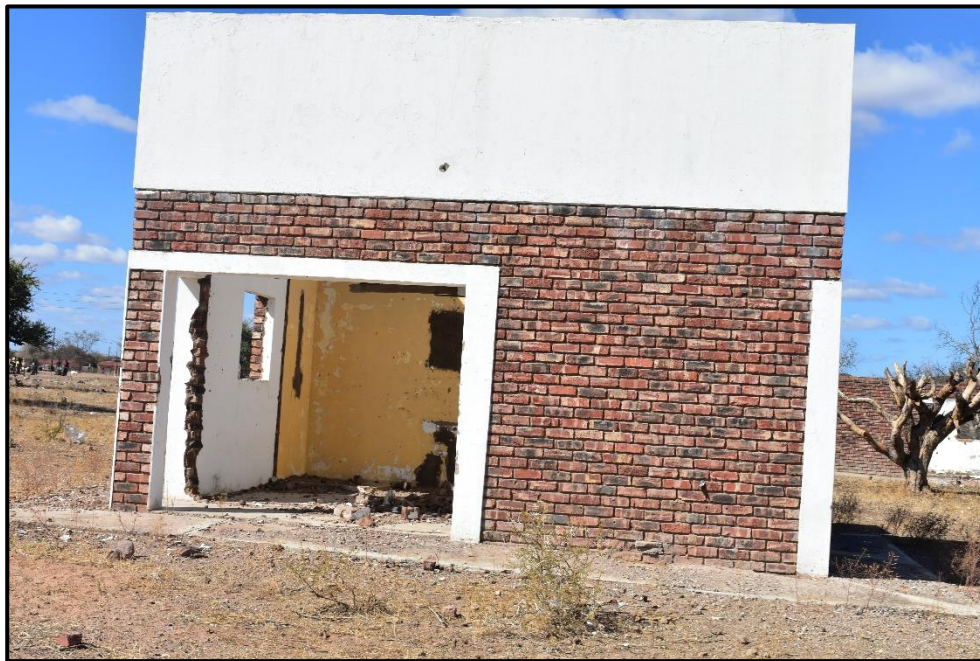
Figure 7: One room dilapidated structure.
