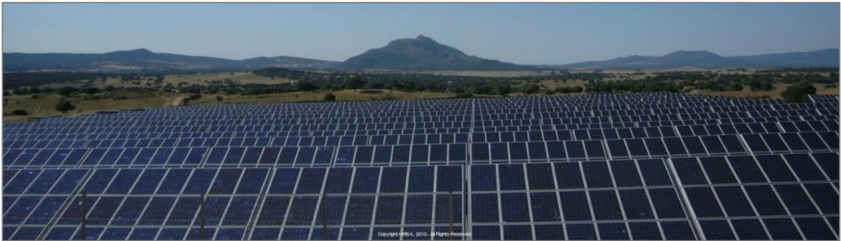
Figure 3: Photograph example of solar panels (Source: www.hawaiirenewableenergy.org/Villamesias2 )
