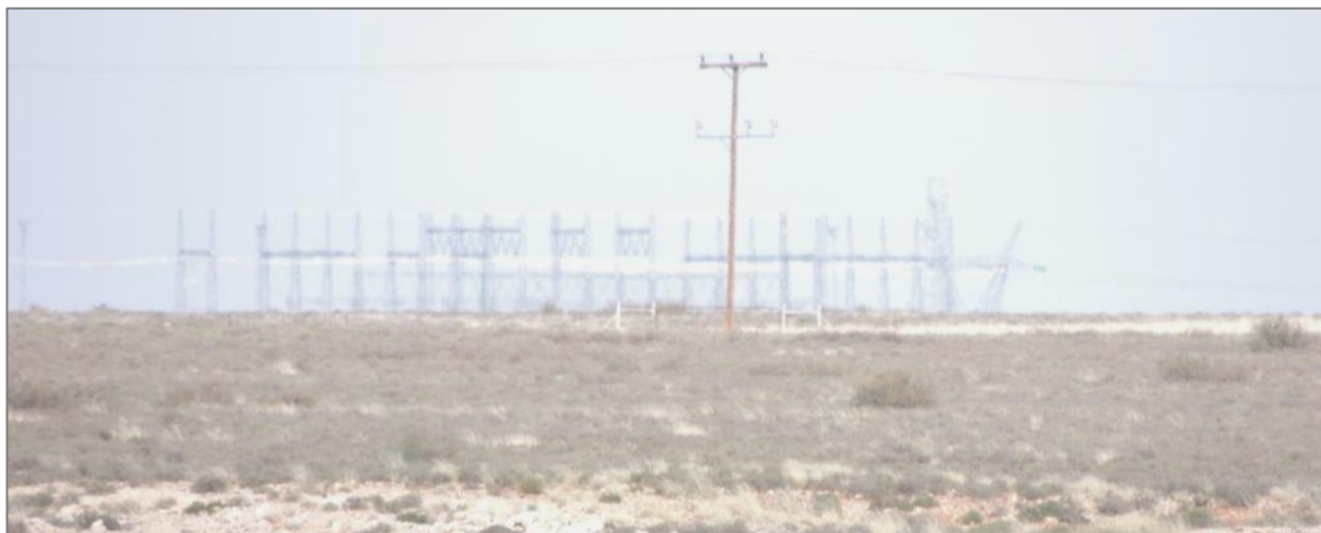
Figure 11: View of existing Cuprum substation
