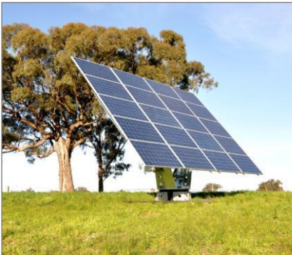
Figure 4: Example of tracking PV solar panels (Source: www.solar_tracker16.ecoforlife.com.au )
