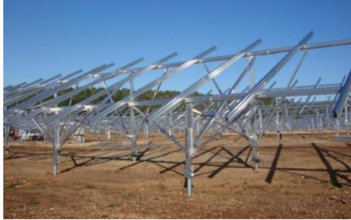
Photograph of an example of PV mounting (Source: VRMA)
