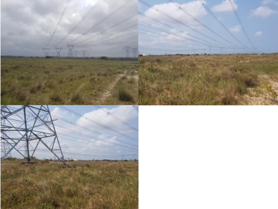
Figure 21: Existing Powerlines in the interaction of East-West Study Area and East-North Study Area
