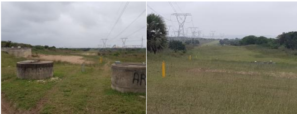
Figure 16: Water infrastructure and servitude along the existing Powerlines and west of the Transnet railway line
