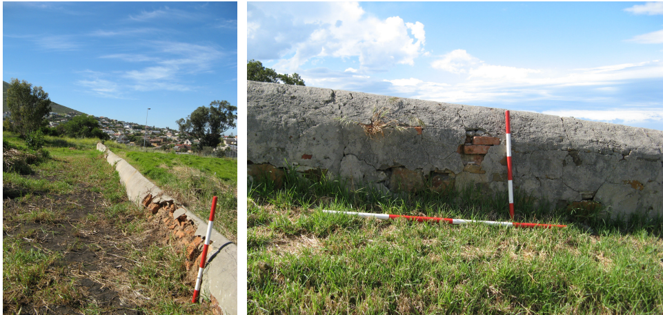
Figure 26: Two repair episodes to the southern section of the wall, both dating to the 19 th century. The image on the right shows typical early 19 th century baked brick, identified by the thinness of the brick.
