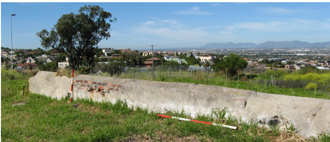
Figure 25: Evidence of modern repair to the werf wall. The werf wall stops just beyond the metre stick, possibly having been demolished when the ruins of the granary/kraal complex were flattened. Along this wall are a number of shallow buttresses.
