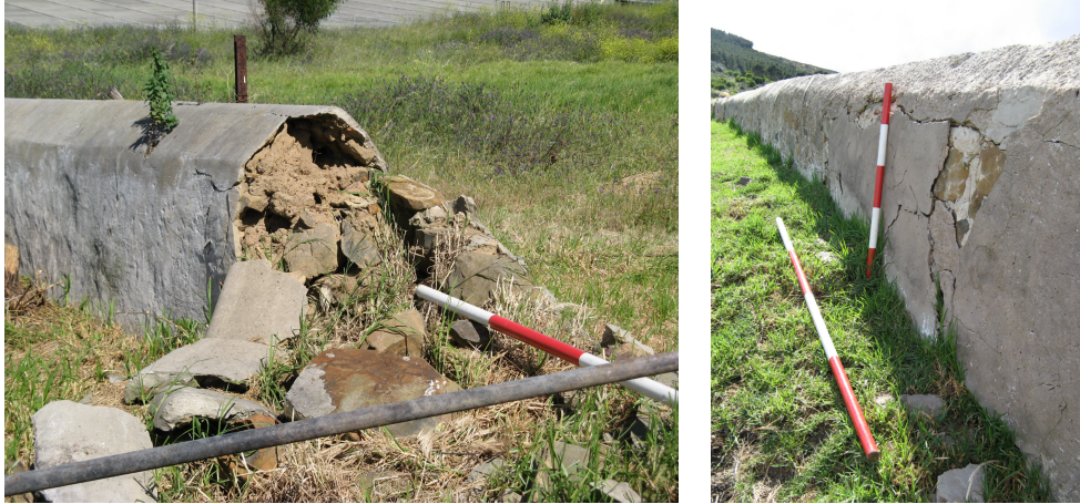
Figure 23: Western portion of the werf wall is the oldest remaining portion of the wall, being stone build with an unbaked brick coping. Shell lime plaster is visible on the exterior part of the wall.
