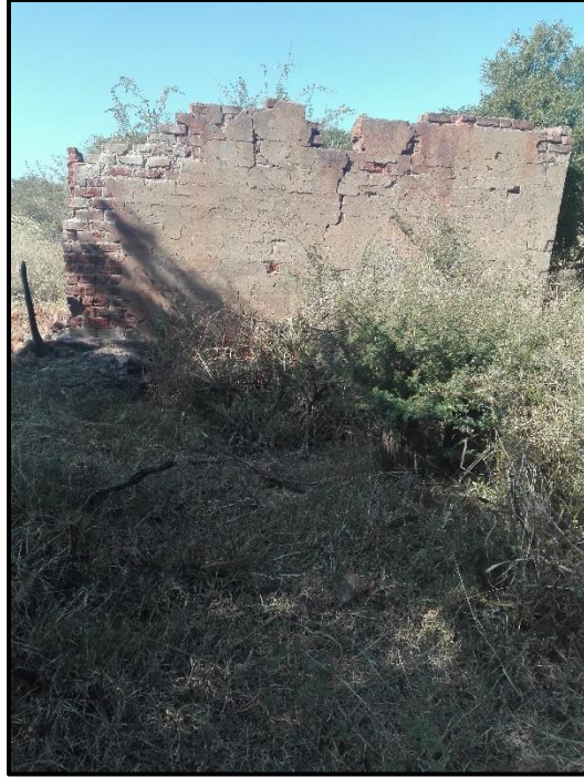
Figure 8: Dilapidated structure in Pella before split of Alternative Corridor 1 and Alternative Corridor 2 line.
