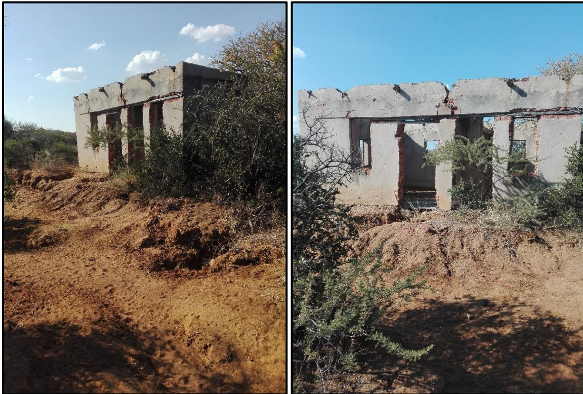
Figure 9: Dilapidated house towards splitting of Alternative Corridor 1 and Alternative Corridor 2 line.
